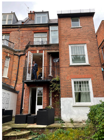
Rear elevation showing non-original first floor extension to the rear bay window
