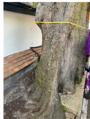
Base of tree T11 as viewed in a westerly direction showing limited planting pit against structure to south
