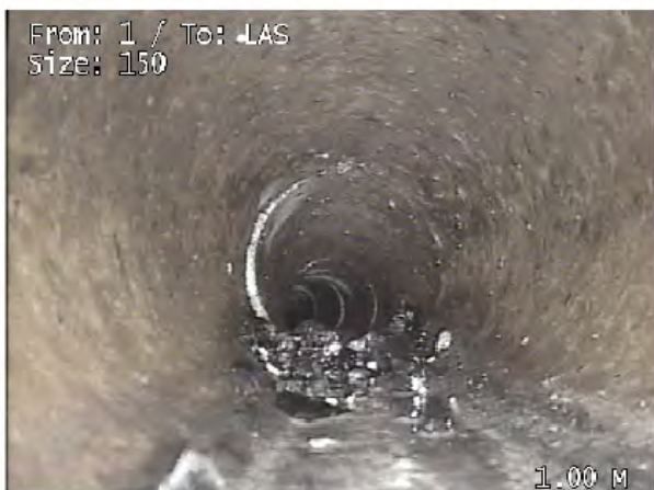
Settled deposits coarse 15% cross-sectional area loss, Start
