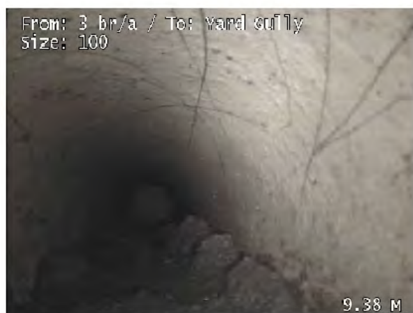
Settled deposits coarse 25% cross-sectional area loss, Start
