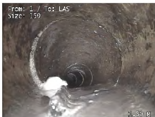
Attached deposits, encrustation at 5 o'clock 10% cross-sectional area loss
