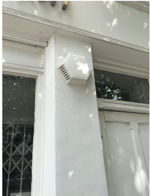
08: Existing Intruder Alarm
