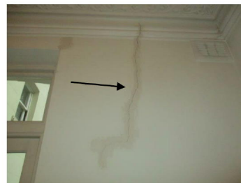
Cracking in ground floor dining room
