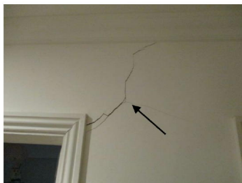
Cracking in basement hallway
