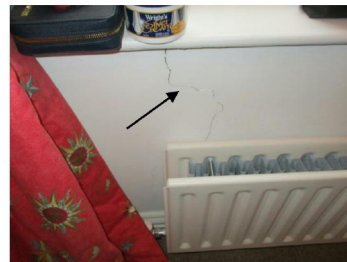
Cracking in upper flat rear study
