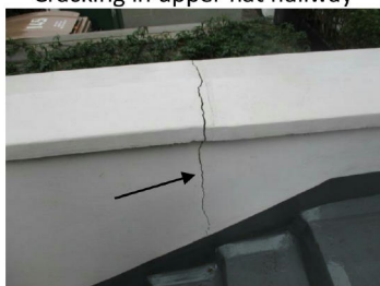
Cracking to front left hand steps boundary wall
