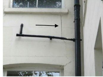
Cracking to rear elevation
