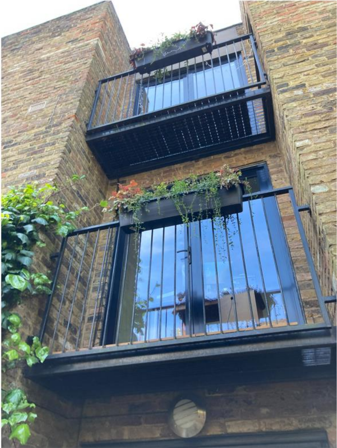
Existing 1 st and 2 nd floor rear balconies (the 1 st floor balcony would be slightly enlarged – to become flush with the 3 storey bays)
