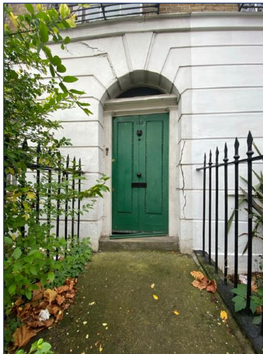
Figure 3- Photograph showing condition of front door
