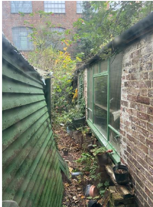
Figure 4- Photograph showing condition of existing rear outrigger and outbuilding
