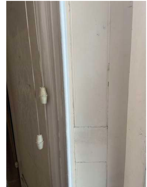
Front Room - original panelling and architrave to front windows - windows are replacement
