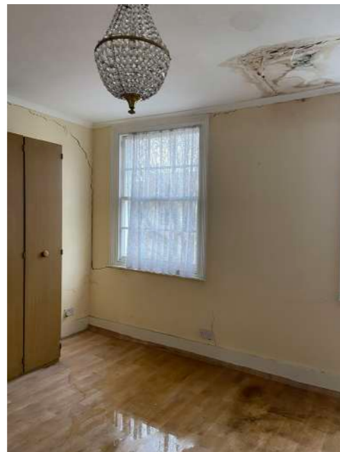
Front Room - showing significant cracking, adjacent to No. 127 Albert Street and historic water
