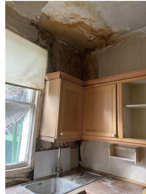
Rear Reception Room - significant damage to existing cornice from historical water damage
