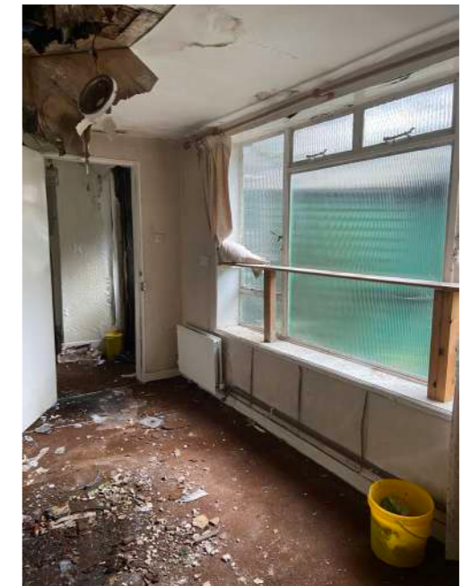
Outrigger - 20th Century Outrigger in complete disrepair
