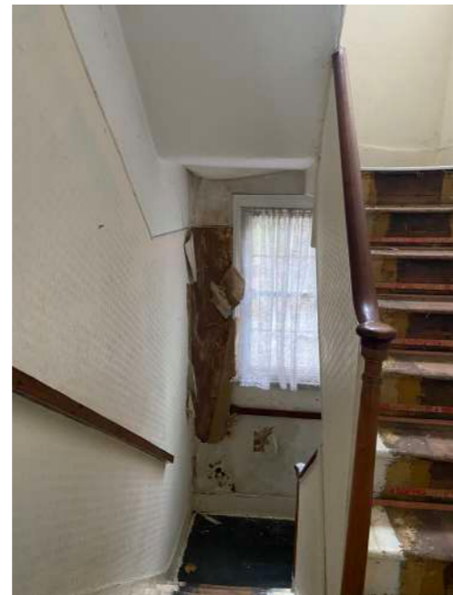
First Floor Landing - looking down to original window. Original stairs with cladding to balusters
