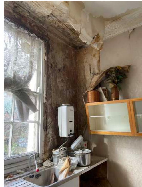
Rear Room - damaged cornice from historic water damage
