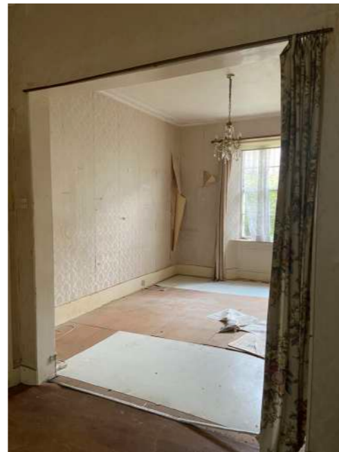
Front Reception Room -view from Rear Reception Room through to Front Reception Room
