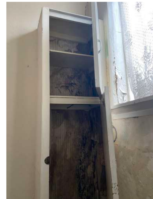
Stairs - later addition cupboard to stair return, showing historic water damage
