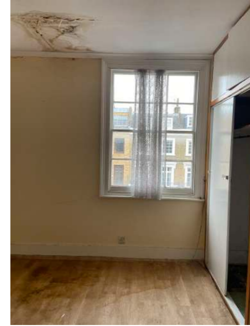
Front Room - view to front, showing water damage and modern cornice
