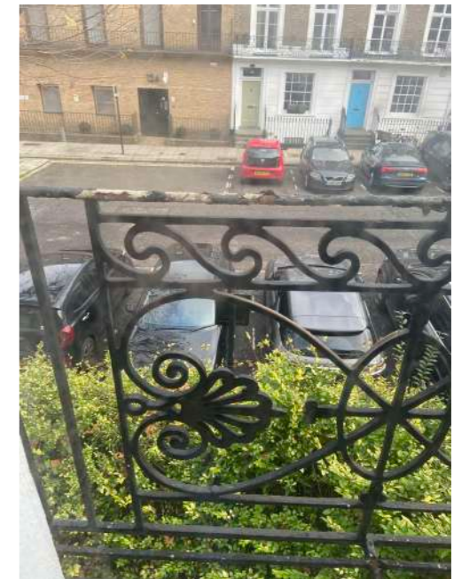
Front Room - view out to metal balconies requiring repair and making good
