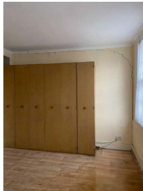
Front Room - showing significant cracking, adj. to No. 127 Albert Street and historic water damage and partition to left hand side
