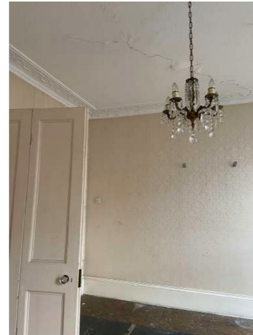
Front Room - significant cracking to ceiling and sloping to floor
