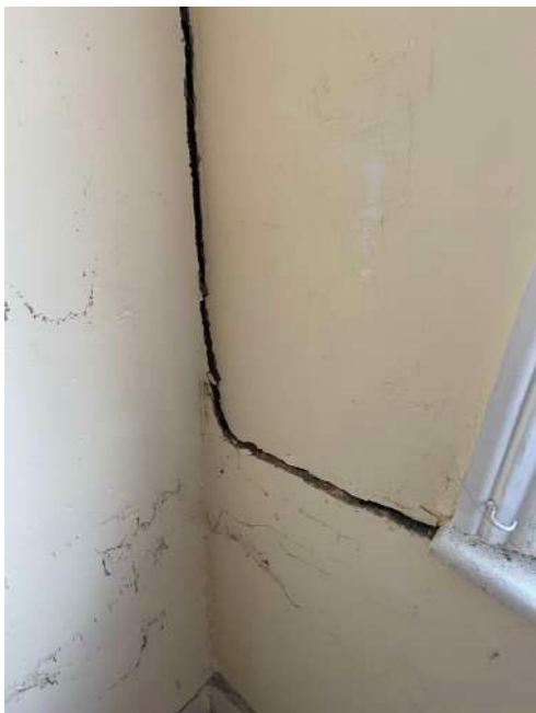
Front Room - showing significant cracking, adjacent to No. 127 Albert Street
