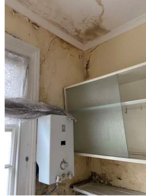
Rear Room - view to rear showing water damage to ceiling and modern cornice
