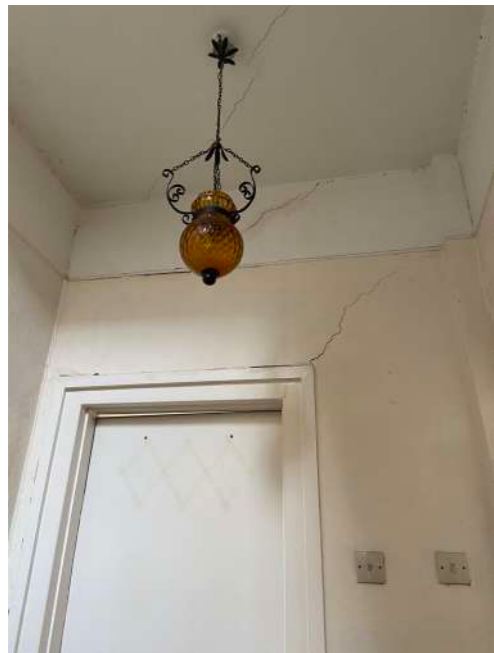
First Floor Landing - significant cracking to walls and ceiling
