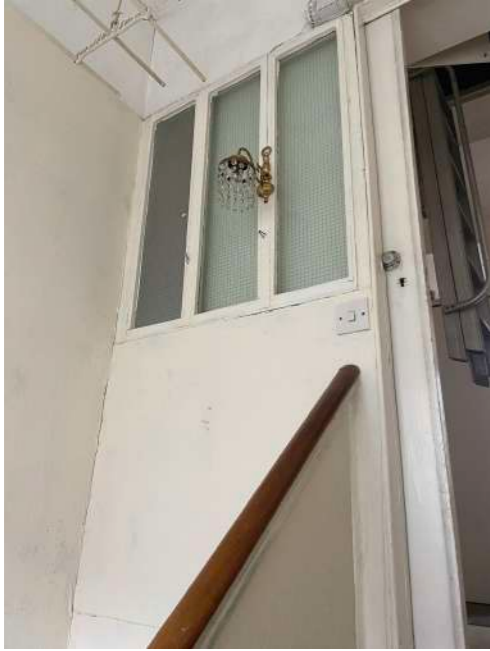
Stairs/Landing - looking up to Second Floor, original handrail removed to allow for partition
