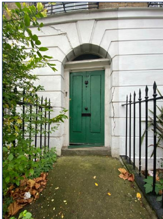
Figure 3- Photograph showing condition of front door
