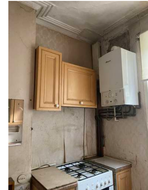
Rear Reception Room - significant damage to existing cornice, pipework and boiler/flue outlets
