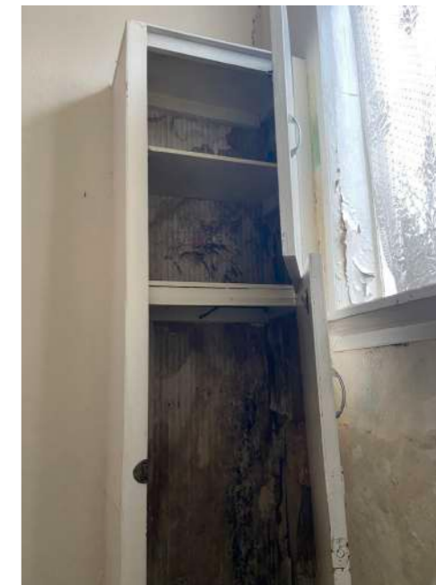
Stairs - later addition cupboard to stair return, showing historic water damage
