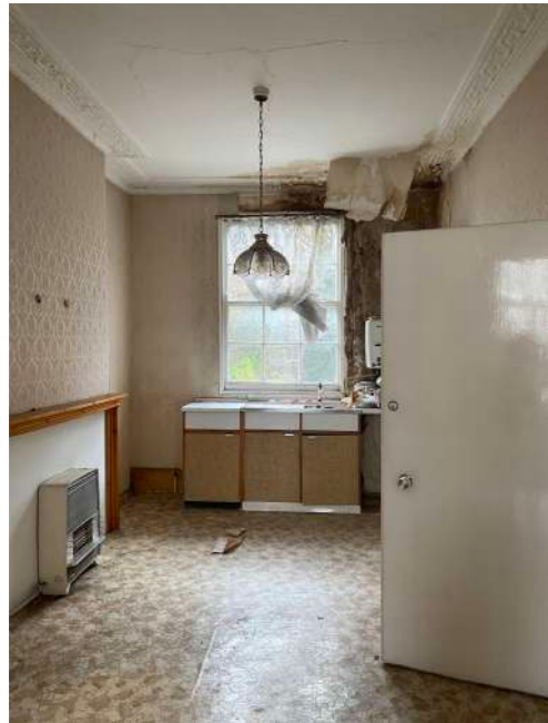
Rear Room - damaged cornice from historic water damage, original doors overlaid and chimney
