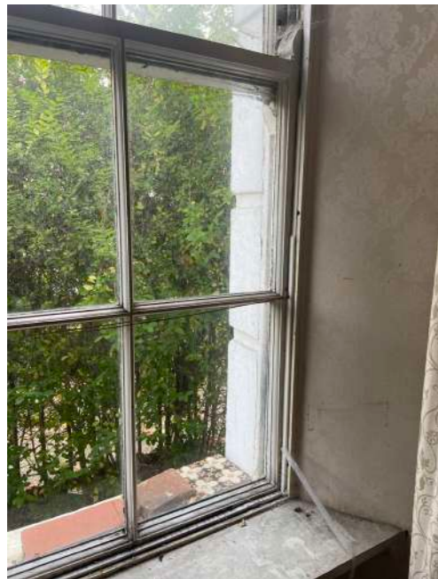
Front Reception Room - single glazed replacement sash windows, style not in keeping with property period
