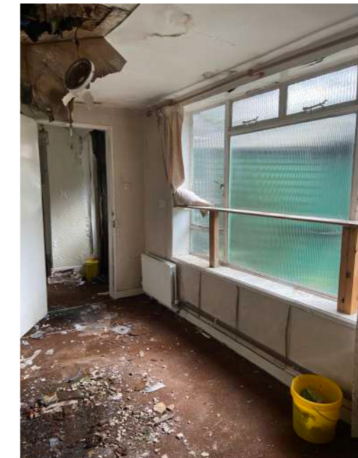
Outrigger - 20th Century Outrigger in complete disrepair
