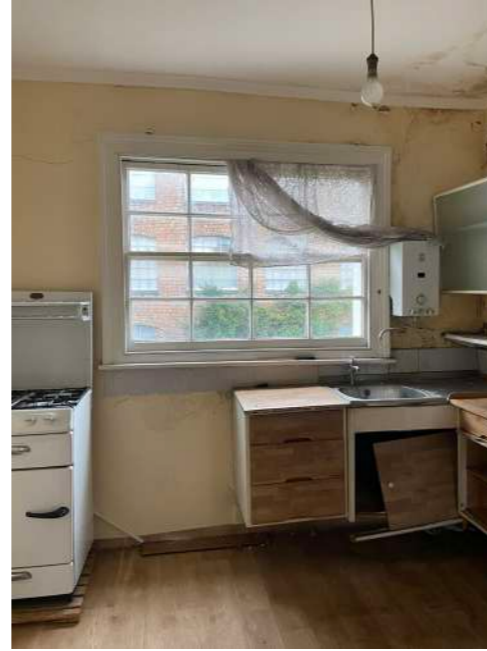
Rear Room - view to rear showing rebuilt facade and window and water damage to ceiling
