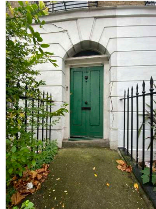
Existing Entrance and Stucco showing cracking
