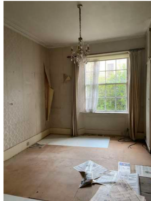
Front Reception Room - significant sloping floor, replacement windows and original doorway
