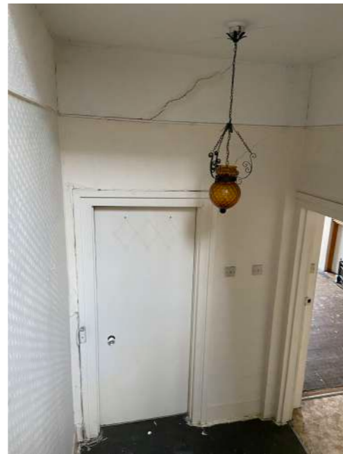
First Floor Landing - looking down to first floor level, significant cracking apparent
