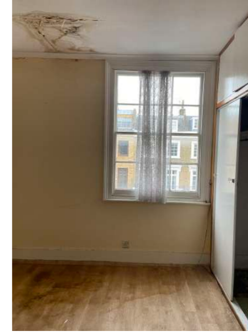
Front Room - view to front, showing water damage and modern cornice
