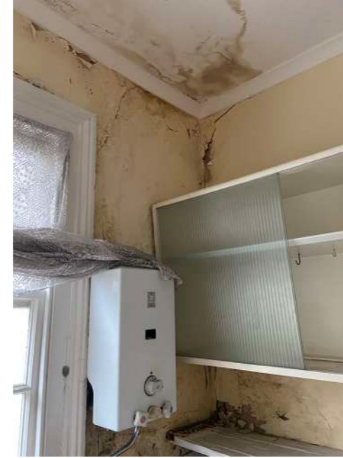
Rear Room - view to rear showing water damage to ceiling and modern cornice
