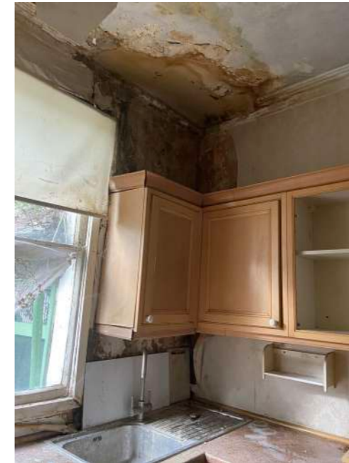
Rear Reception Room - significant damage to existing cornice from historical water damage
