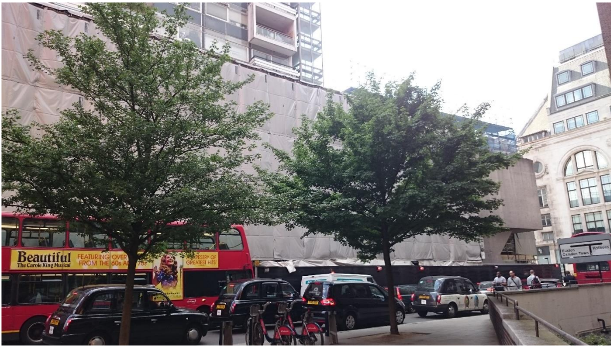
Photo 1 of T3 and T4 looking west
