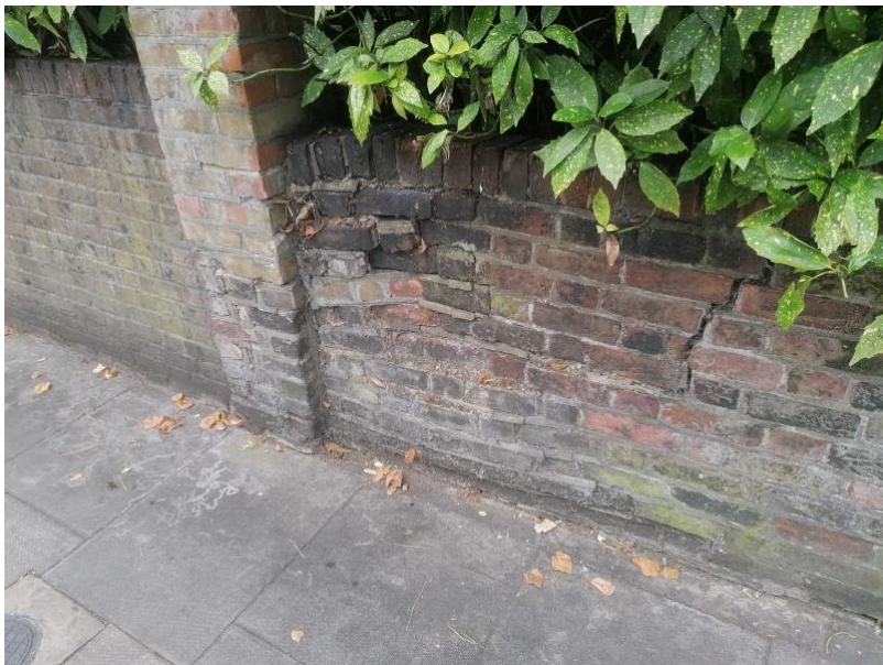
Image 3: damage to wall adjacent to T1.
