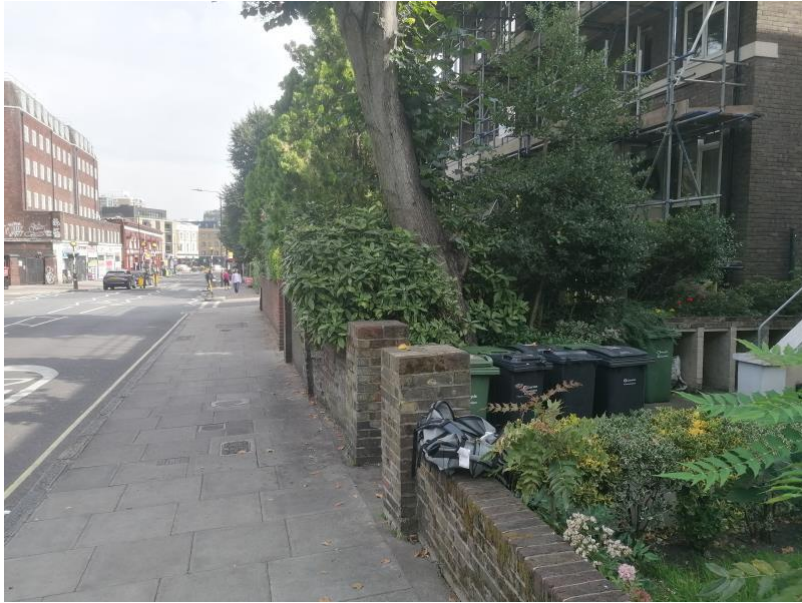
Image 2: stem lean of T1 out towards the road and adjacent boundary wall.
