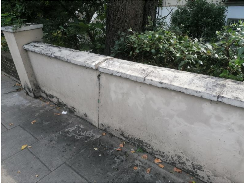
Image 4: movement and damage to wall adjacent to T2.
