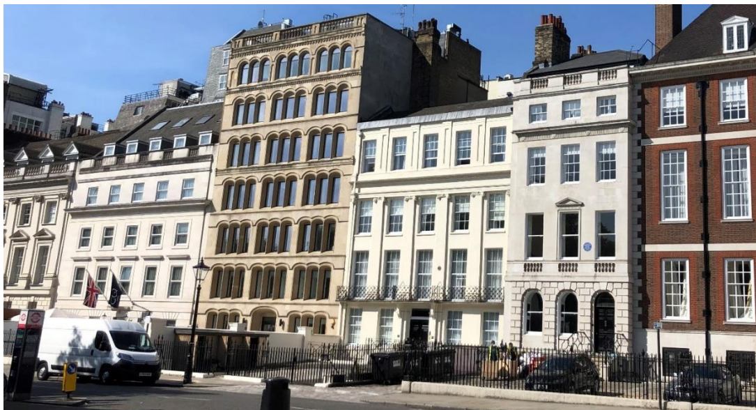
Figure A: No. 64 Lincoln’s Inn Fields with the roof and lead flashing visible.
