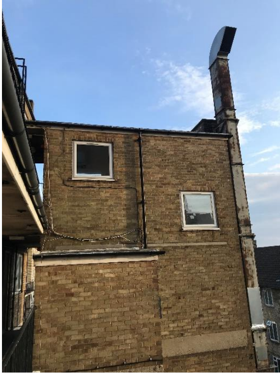
Z Zang Kitchen Flue (taken from the 1 st Floor balcony)
