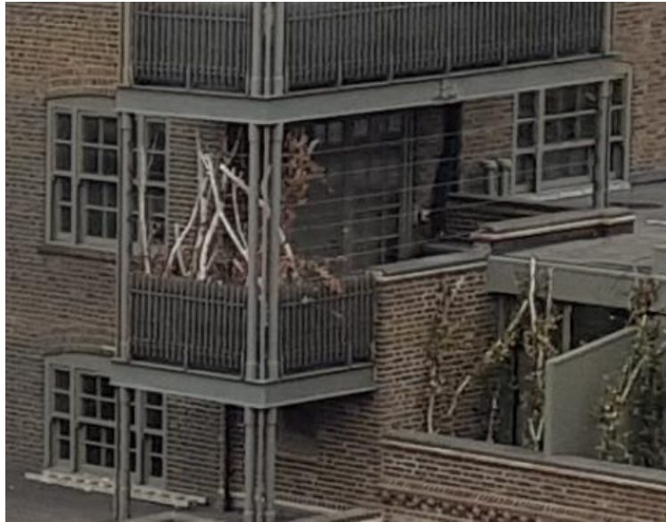
View of the dropped level of balcony at Flat 5 No. 10 Belmont Street
