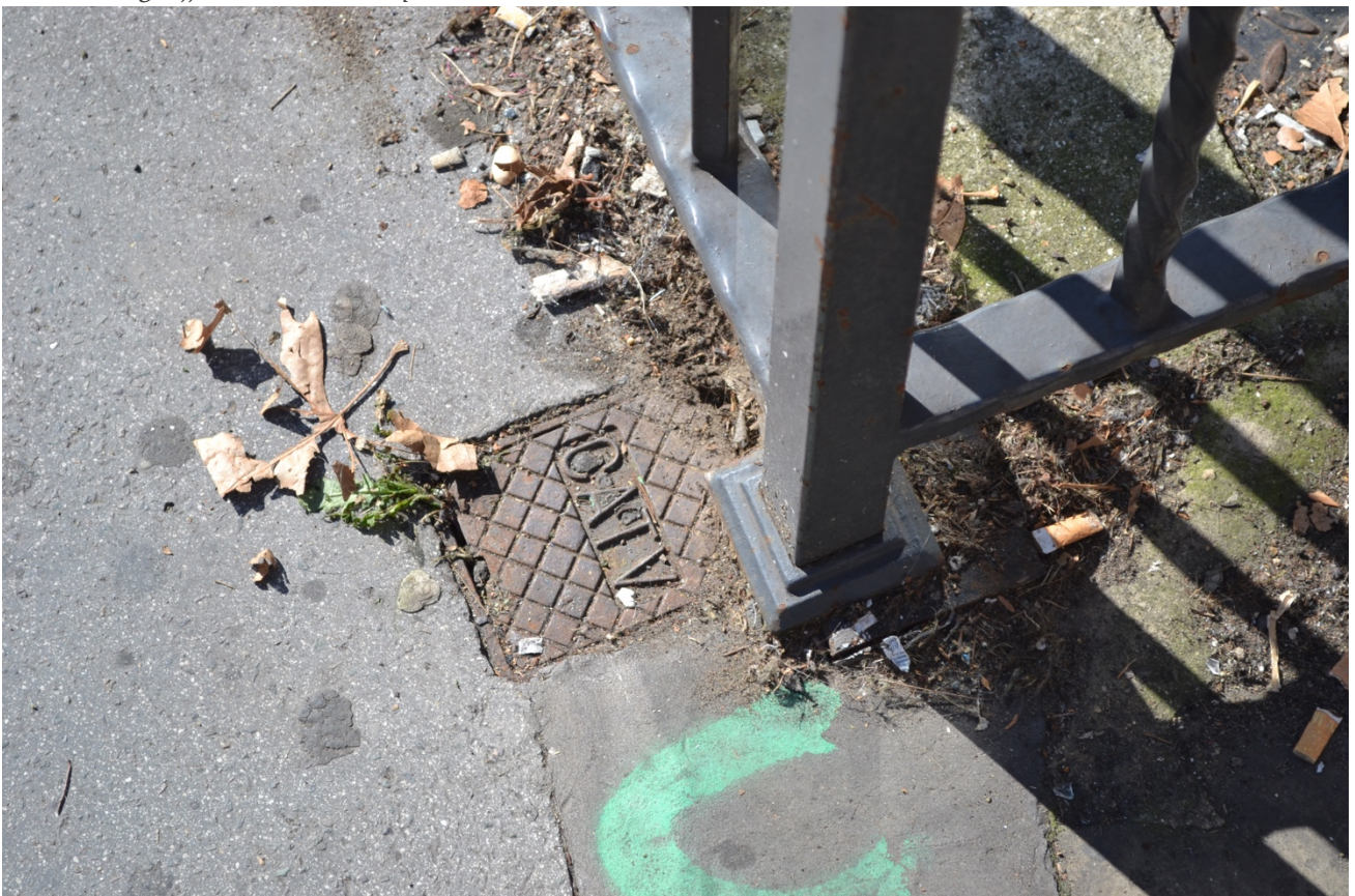
Below: Railings affixed to cable TV inspection cover
