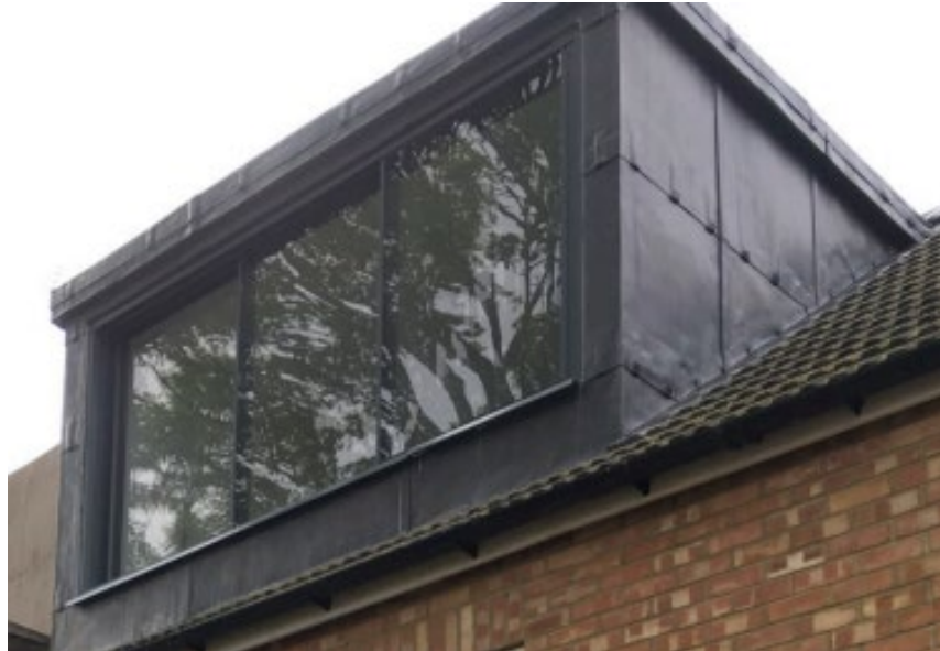
Example of proposed aluminium window frame to be used on mansard roof
