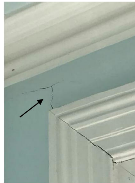
Cracking in bathroom
