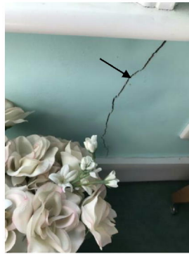
Cracking in bathroom
