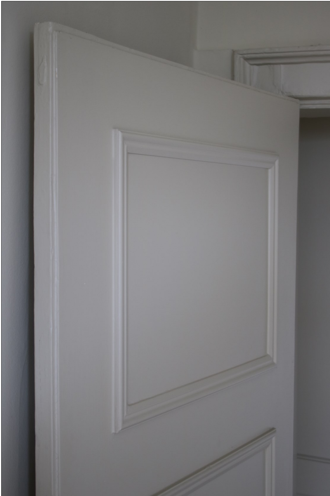
Photograph 6: Interior second floor left hand room door to bathroom -note the planted panelling applied to the earlier door to provide a consistent finish with the bathroom beyond. Note also the earlier frame and architrave indicating an older opening at the top of the picture Photograph =by the author
