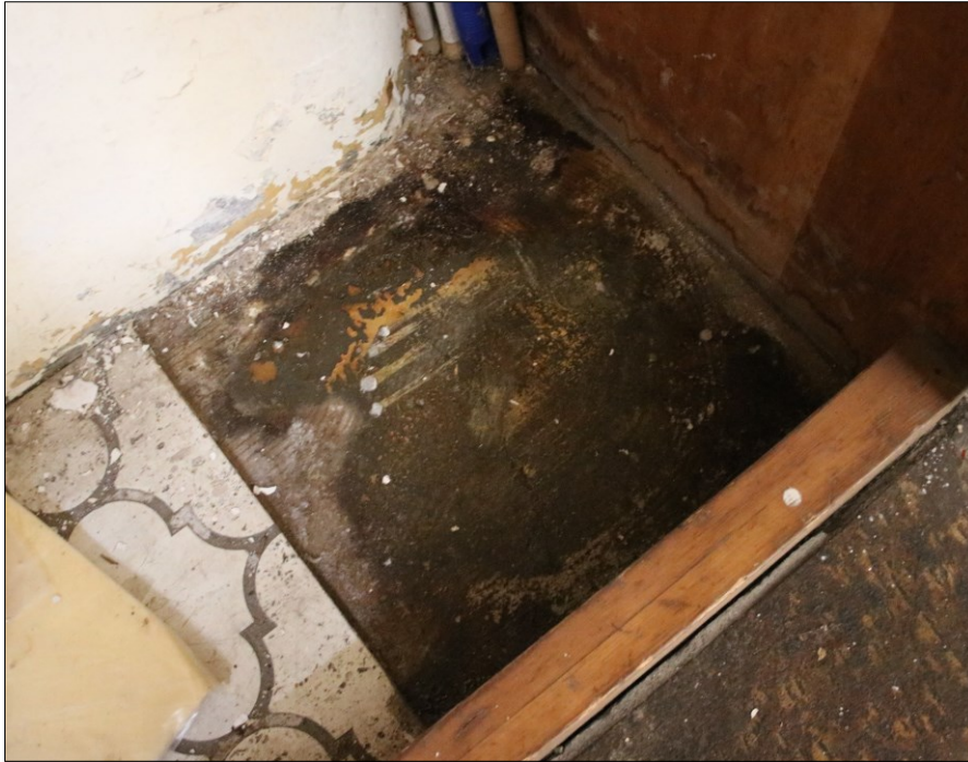
Photograph 7: Detail of basement floor finishes – note the higher level of the current ceramic tile surface, the earlier pale patterned tile covering and the exposed concrete below Photograph by the author
