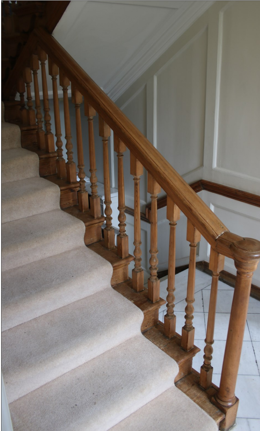
Photograph 2: Stair ground floor flight from hall – note the shallow rise of the treads and the open or cut string with two balusters rising directly from each tread which contrasts with the deeper treads and closed string of the basement flight Photograph by the Author
