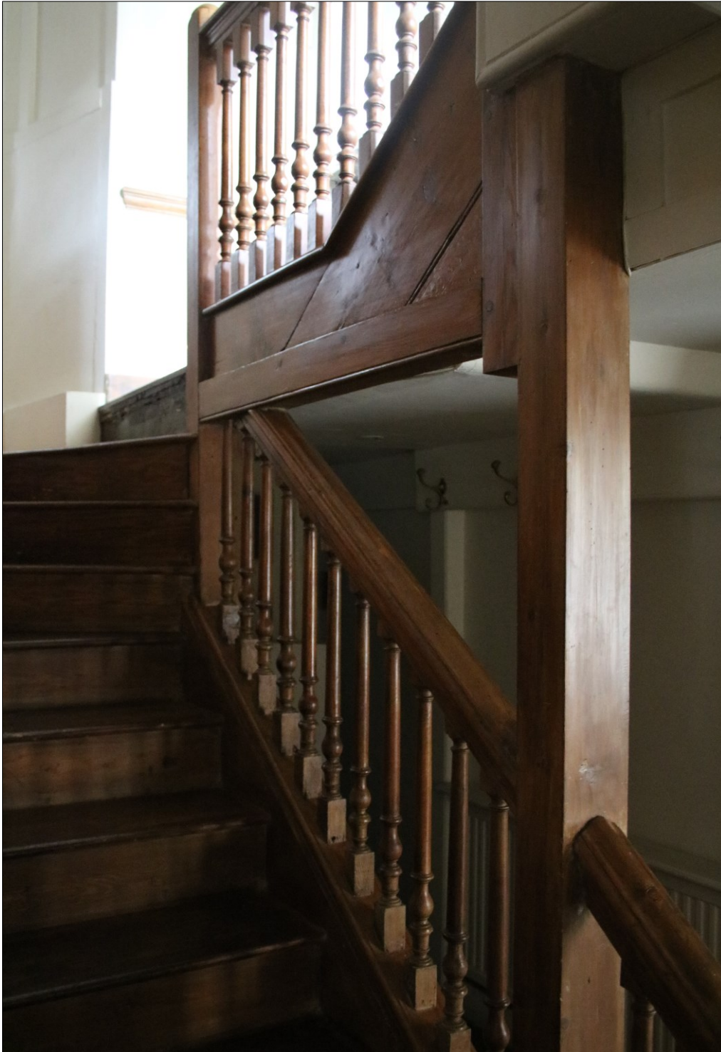
Photograph 1: Stair from basement to ground floor-note the unusually high quality of the materials and balusters for such a humble location. The positioning of the stair either side of the supporting post is also unusual and potentially indications of re-use or adaptation of an earlier grander stair Photograph by the author
