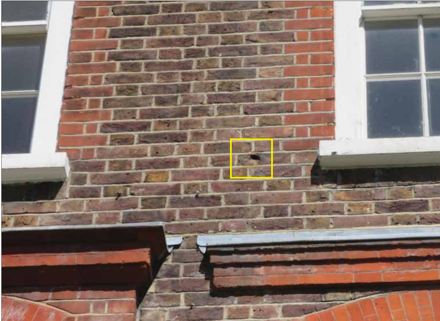
Image 34: Brickwork of the Front Elevation, Relatively Recently Repointed in Cementitious Mortar.
