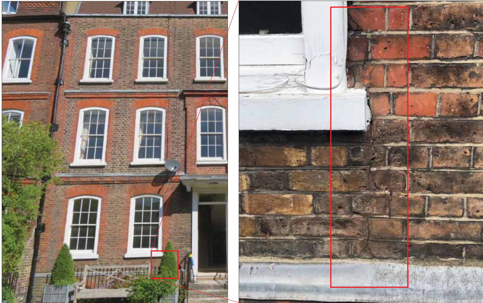
Images 32 & 33: Cracking to One of the Window Openings of the Front Elevation.
