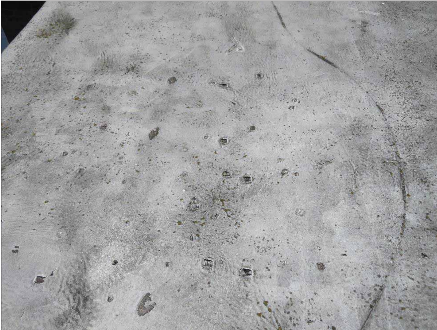
Image 8: Series of Square Puncture Holes to Roof 2.
