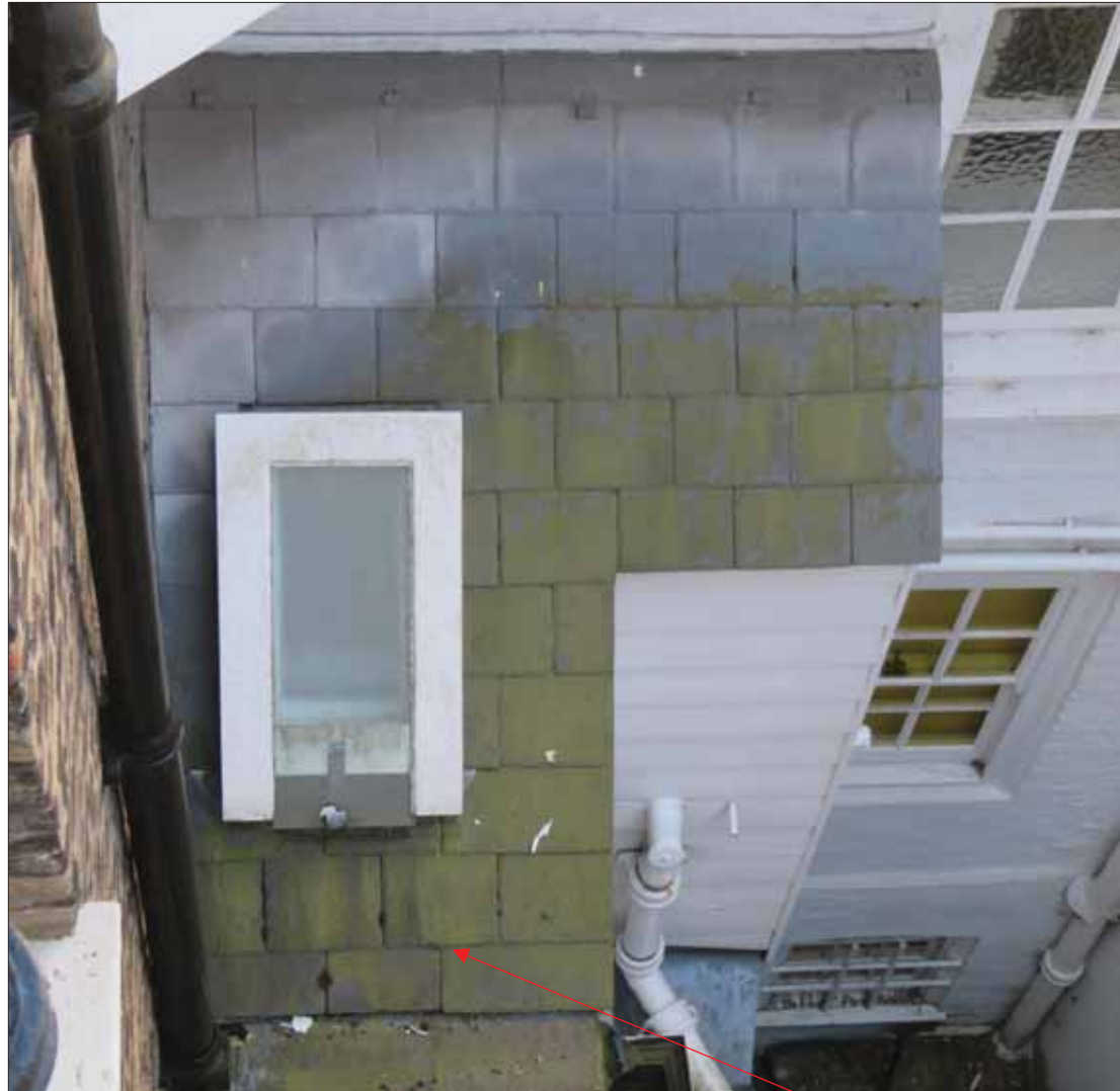
Image 14: Slate Covering of Roof 6 with Single Previous Lead Tingle Repair.
