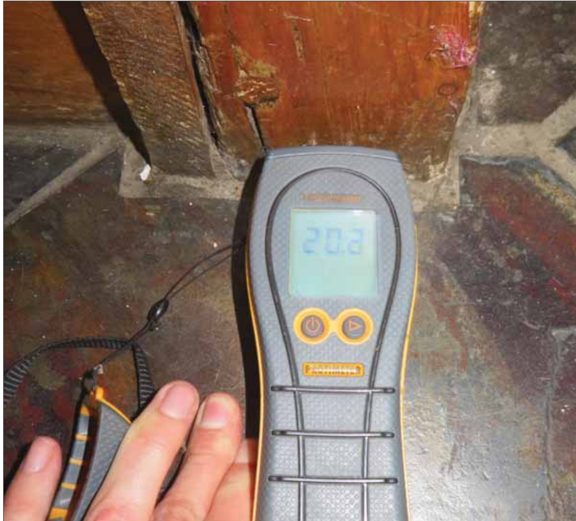
Image 45: Elevated Moisture Contents to the Timbers at the Base of the Staircase.
