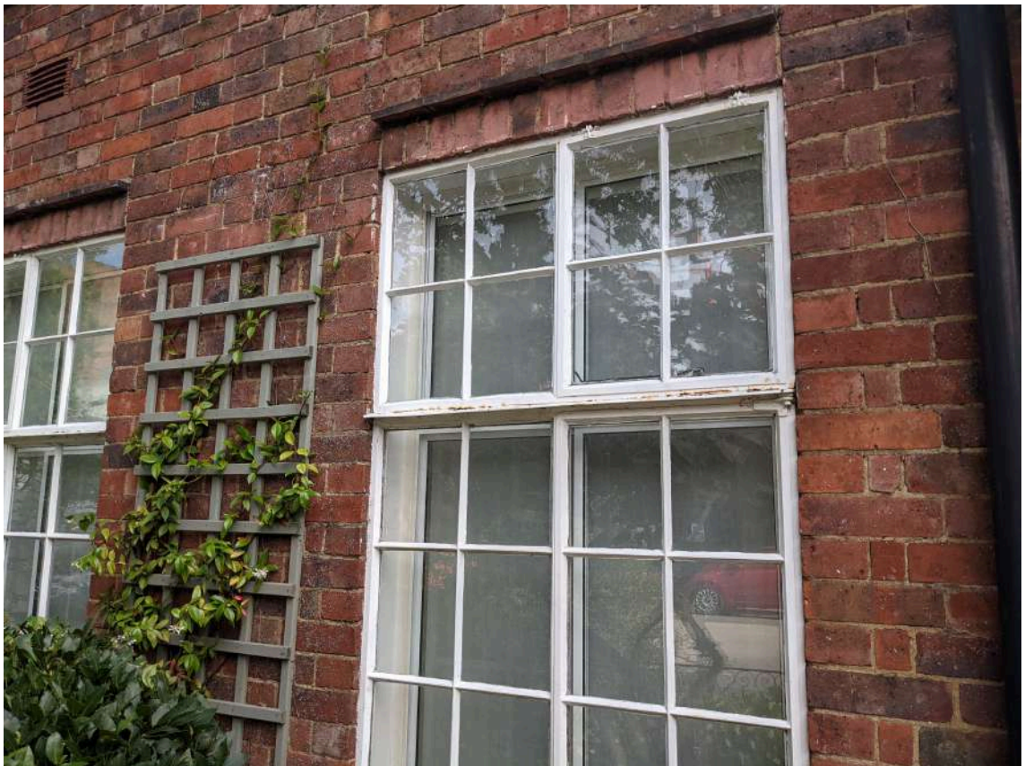
Images of the detail design of the existing glazing to be replaced like-for-like.
