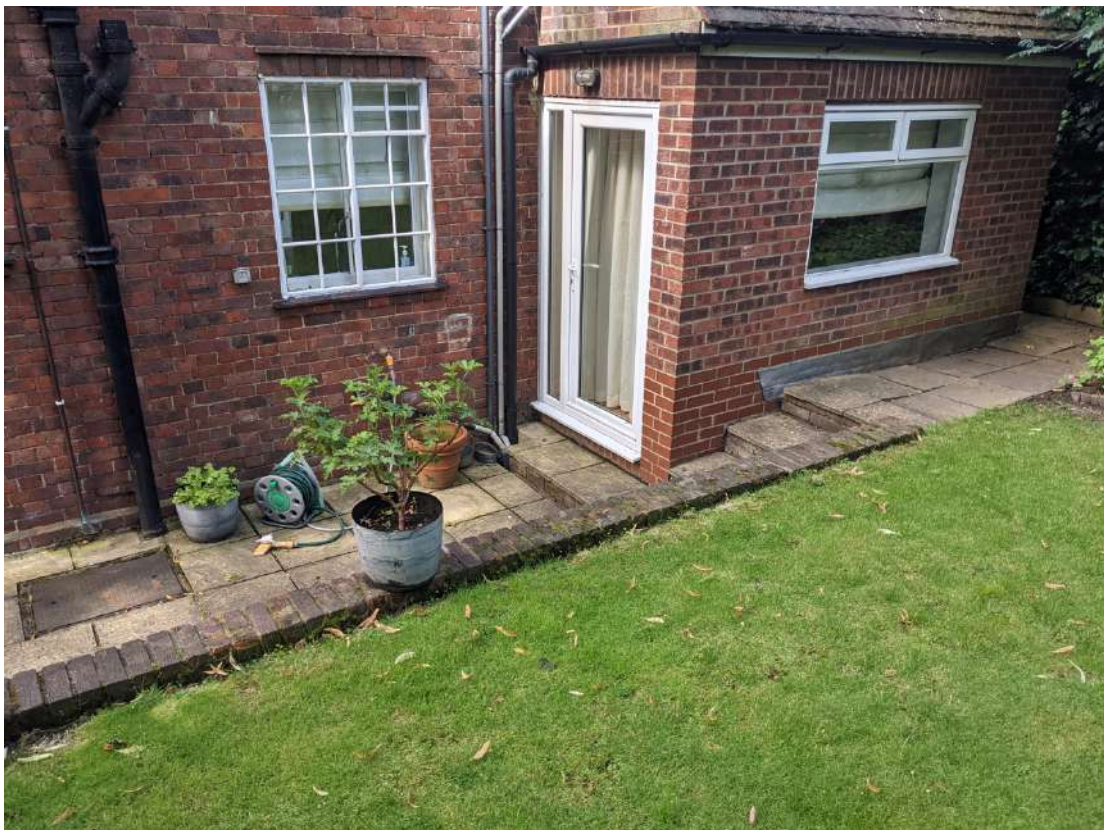
Existing non-original timber and uPVC window and glazed door to be replaced with more sympathetic steel units.
