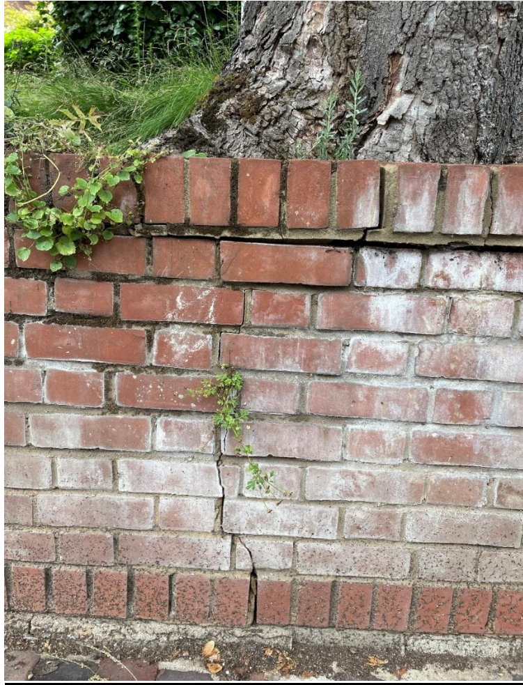
Photo 5 – Cracking at the tree location
