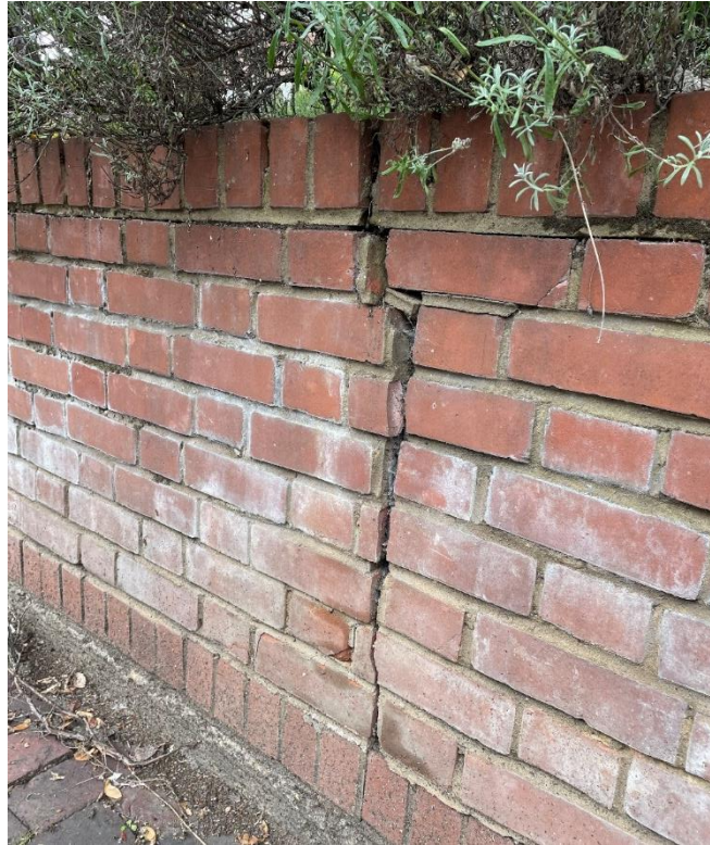
Photo 3 – Vertical tapering crack at approximately 2.4m from the tree towards the driveway
