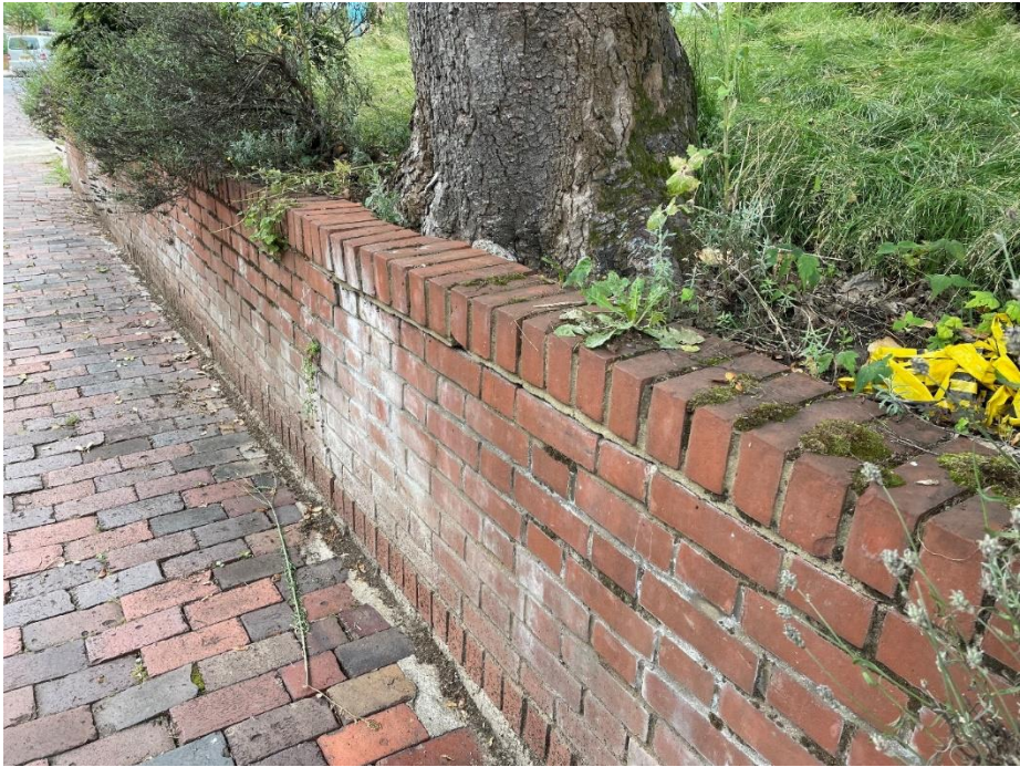
Photo 2 - Leaning wall at tree location
