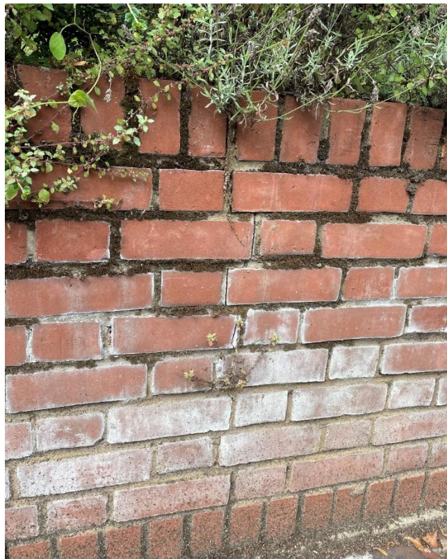
Photo 4 – Tapering vertical crack at about 2.3m the other side of the tree
