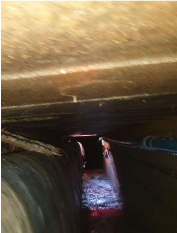
TWO DAMAGED LINTELS FIVE METRES FROM MH3 TOWARDS MH4
