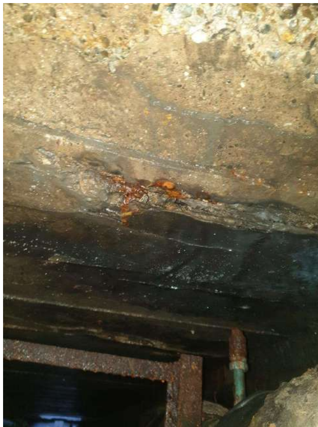
CORROSION BEGINS 2 METRES FROM MH3 TOWARDS MH2
