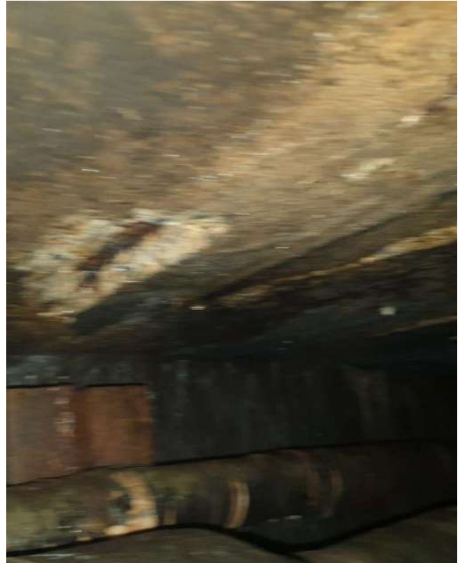
HEAVY CORROSION TO LINTEL ONE METRE FROM MH4 TOWARD MH3
