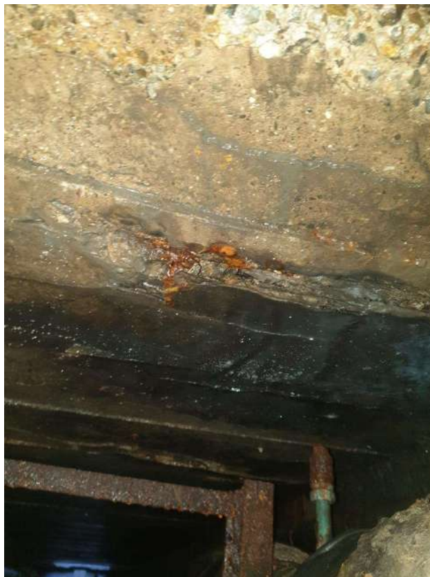
CORROSION BEGINS 2 METRES FROM MH3 TOWARDS MH2
