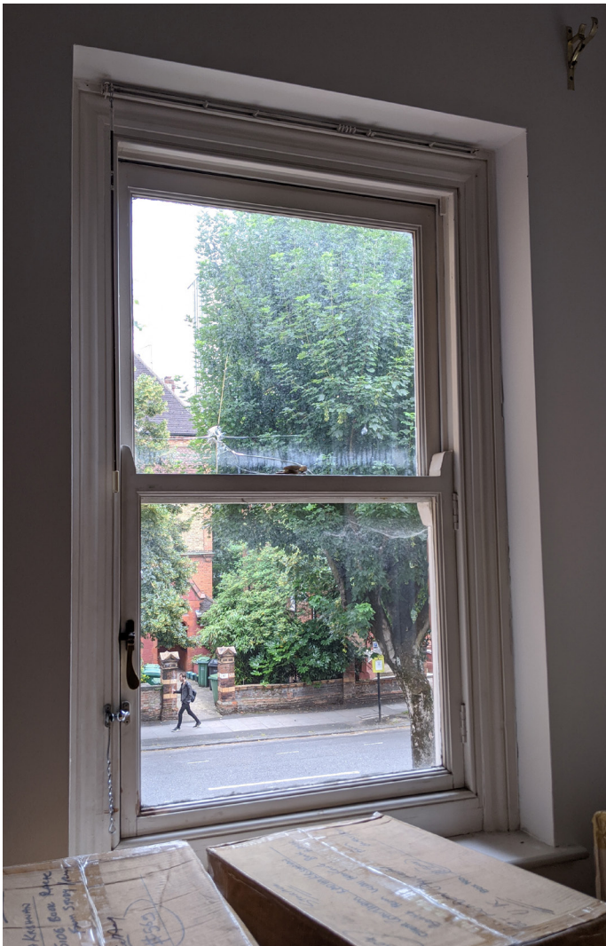
Existing Condition of Windows - note broken glass
