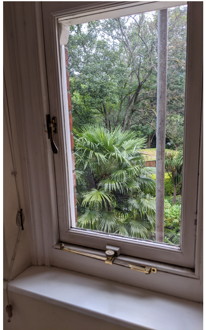
Existing Condition of Windows - casement window to be replaced with sash to match others
