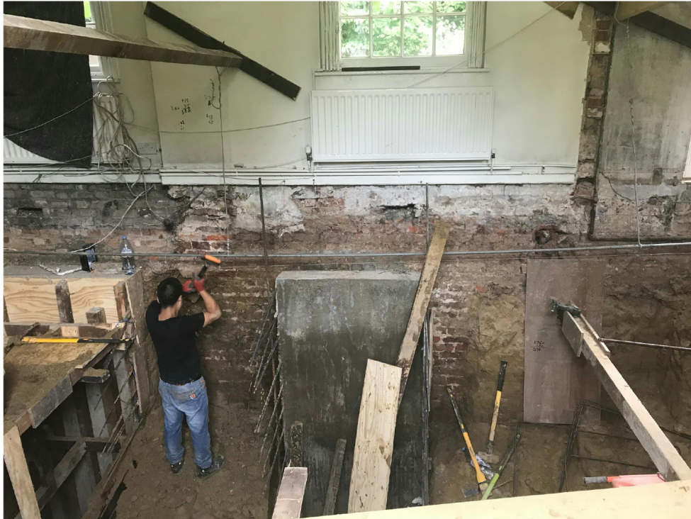
Fig.1 Picture showing basement walls uncovered by removal of back fill. The depth of the walls is clearly far more than any 18 th or 19 th century trench foundation indicating that this was clearly a basement.
