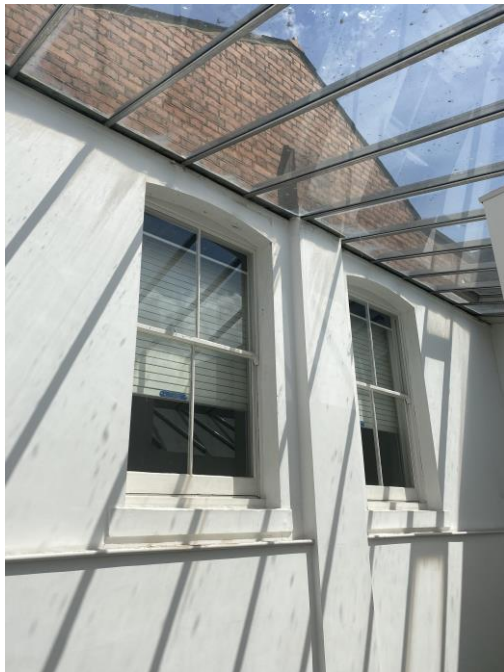
Figure 8: South elevation now rendered over with brick shown about the glazed roof.
