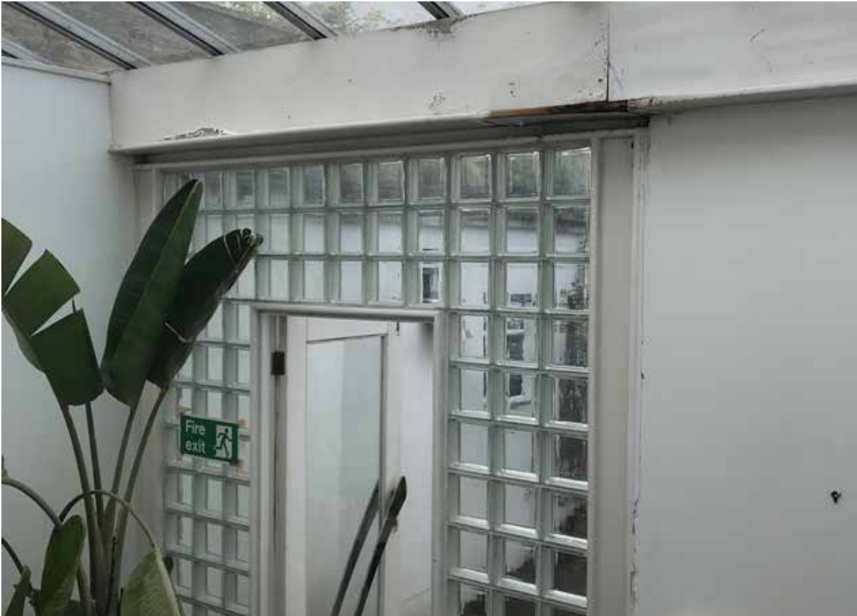
2. Existing lean-to structure with glass block wall showing signs of disrepair
