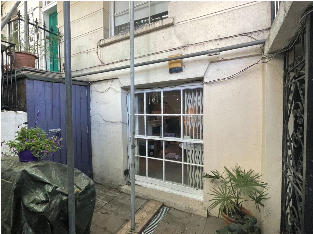
Figure 4 – External view of the window within the living room at basement level
