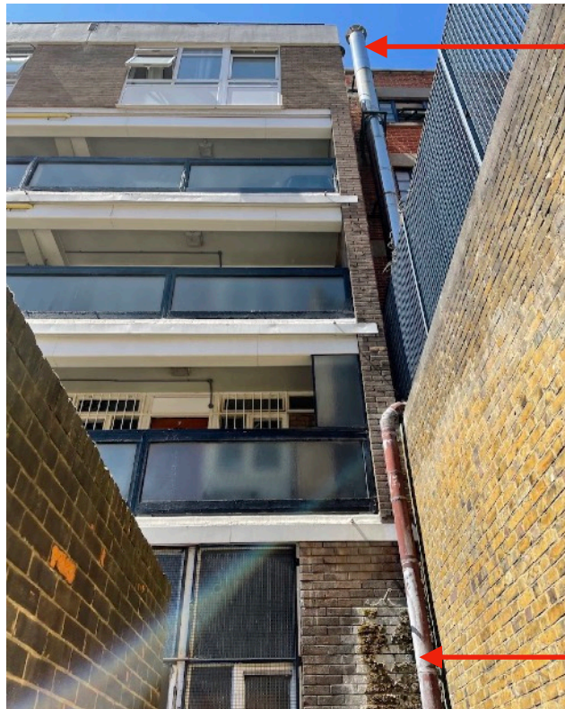
Photo of ducts at rear of the building
