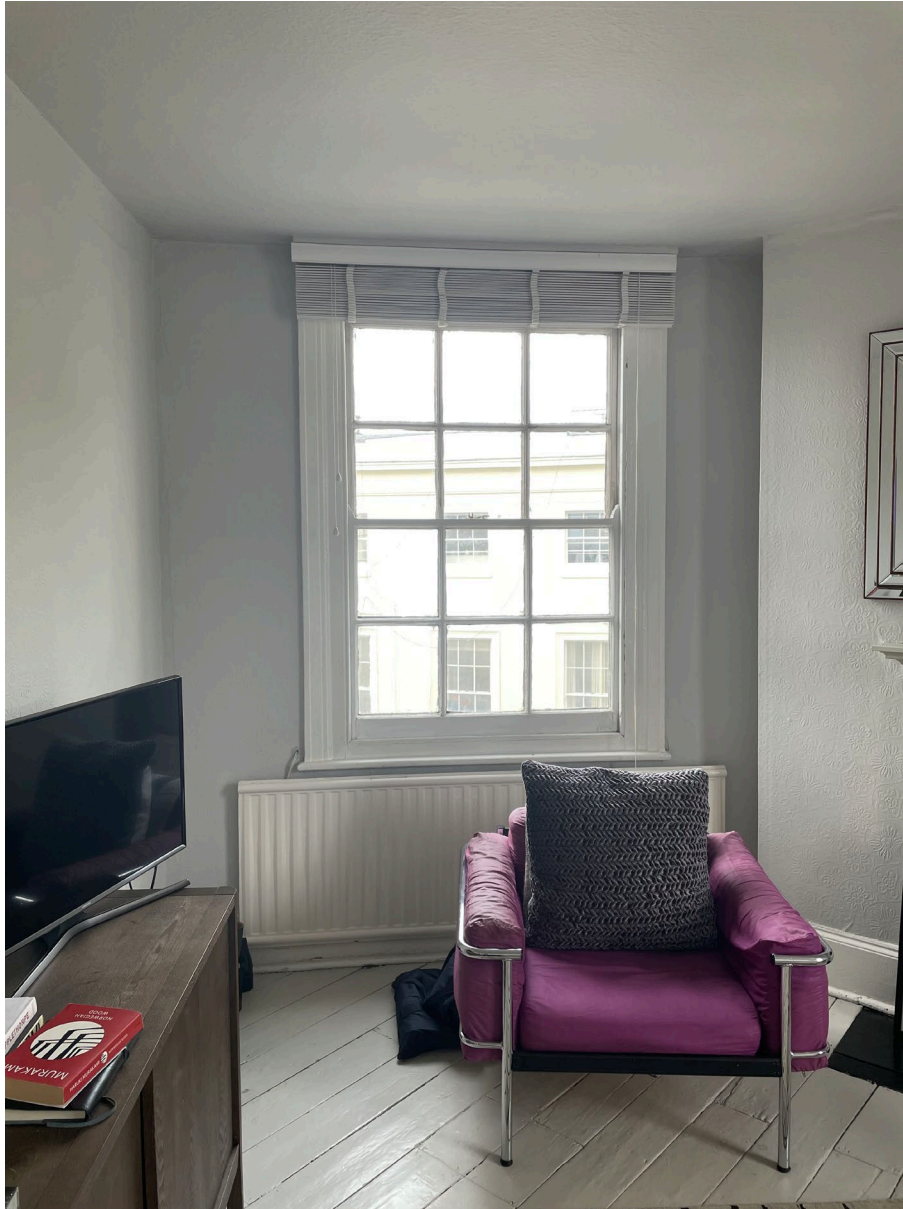
Figure 4: Internal view of left sash window in the living room at second floor
