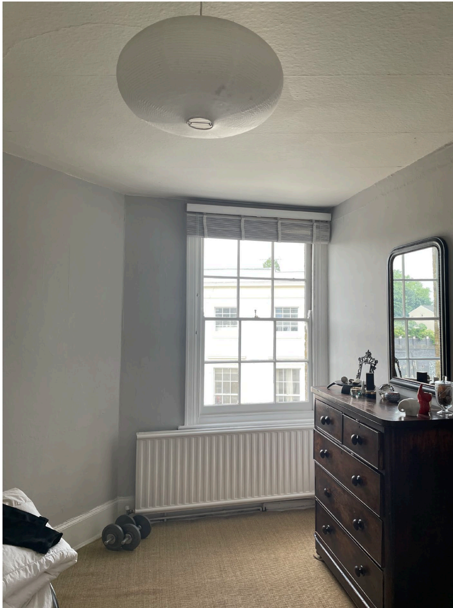
Figure 6: Internal view of sash window in the main bedroom at second floor
