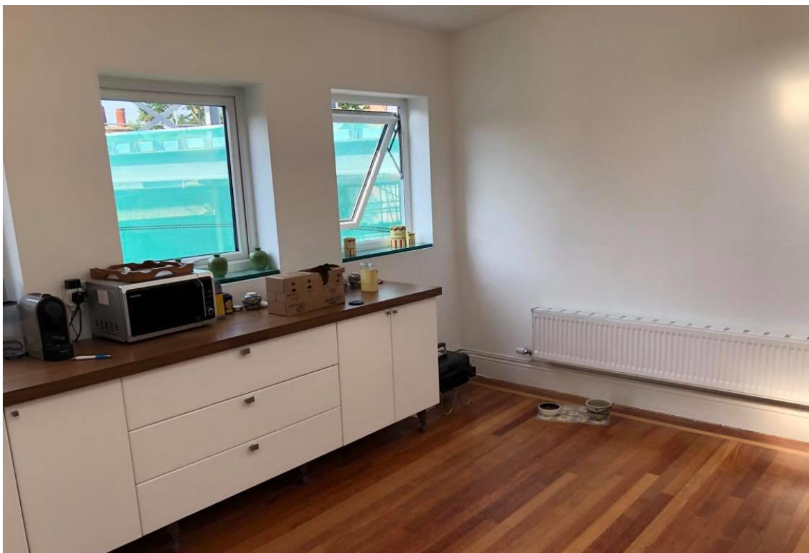
Figure 1.7: View of the East Wall (under construction) from the first floor kitchen and dining room
