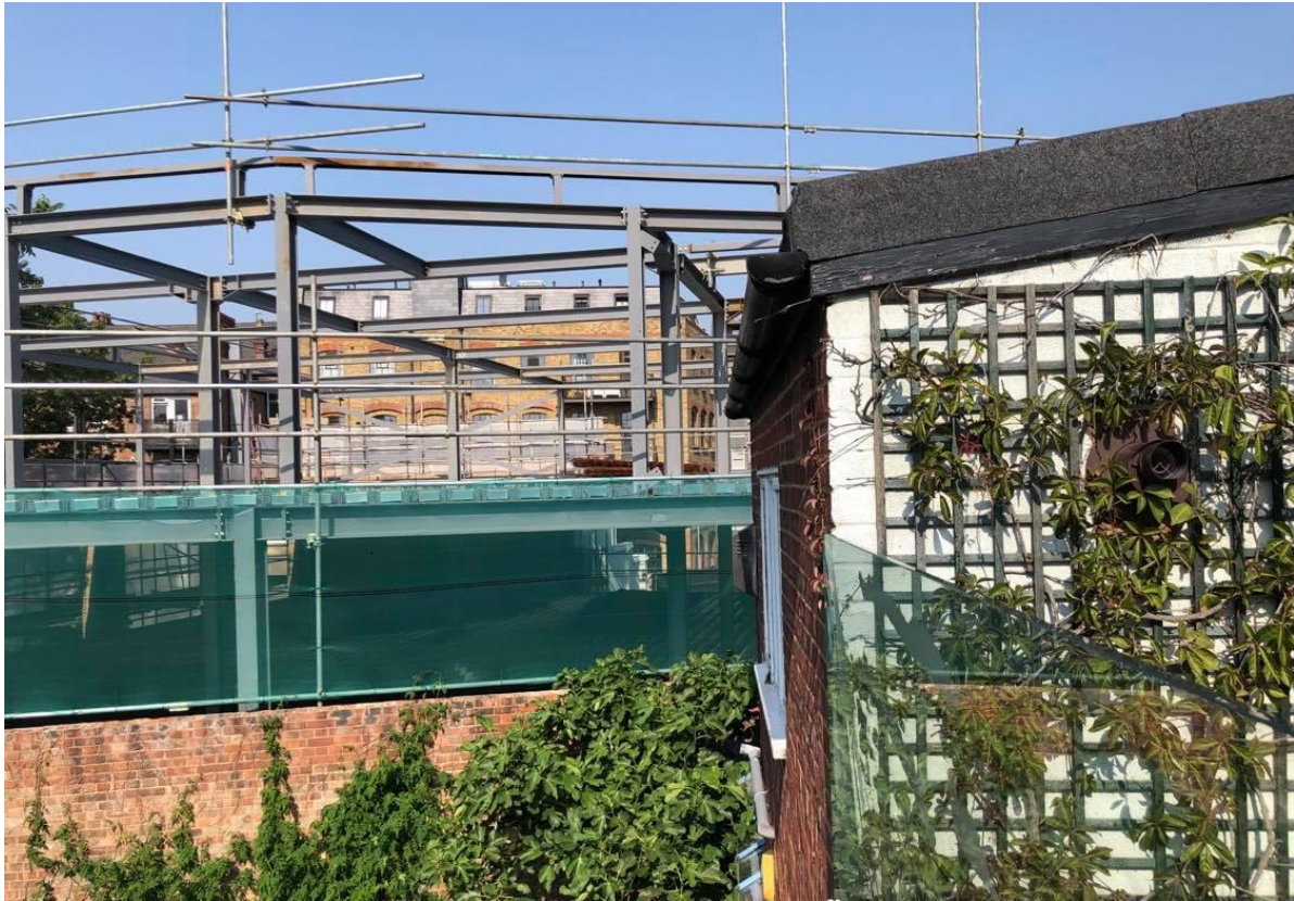
Figure 1.4: View of the East Wall (under construction) from the rear terrace, steel frame above window
