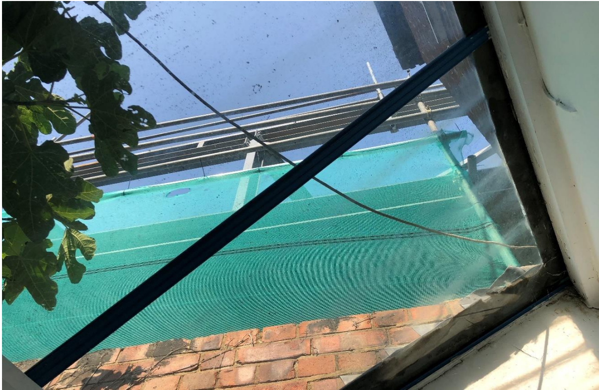
Figure 1.8: View of the East Wall (under construction) from ground floor 'main bedroom'
