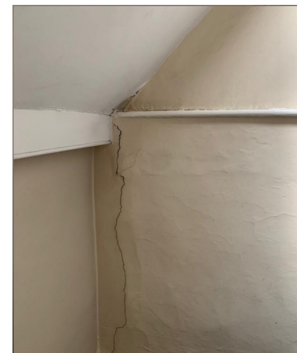
Visible cracking of walls
