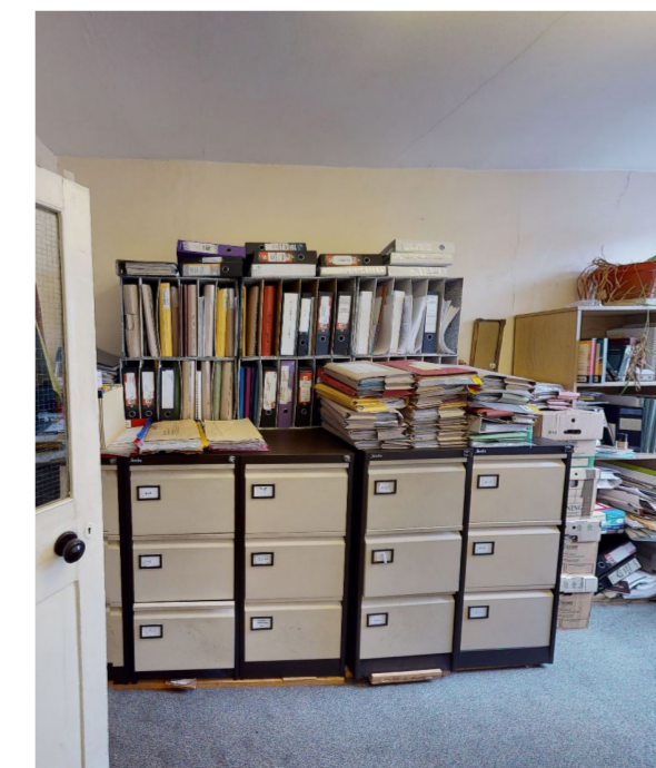
Wooden blocks used to support filing cabinets due to uneven floors
