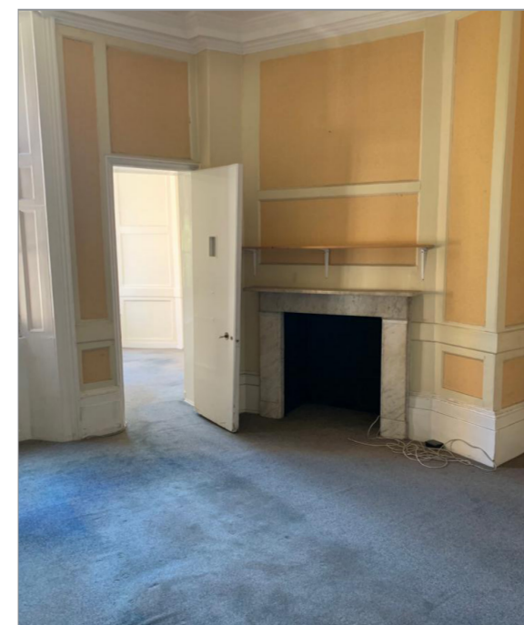
One of the larger office spaces with a maximum warped timber doors and existing panelling
