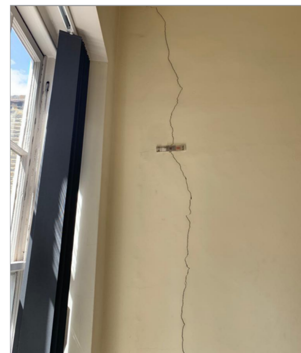
Significant cracking to the party wall within stairwell
