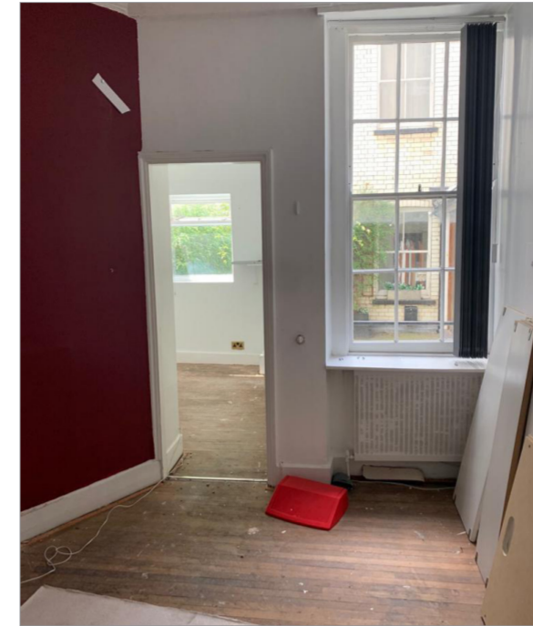
Condition of existing ground floor office space, looking through to non-original rear extension
