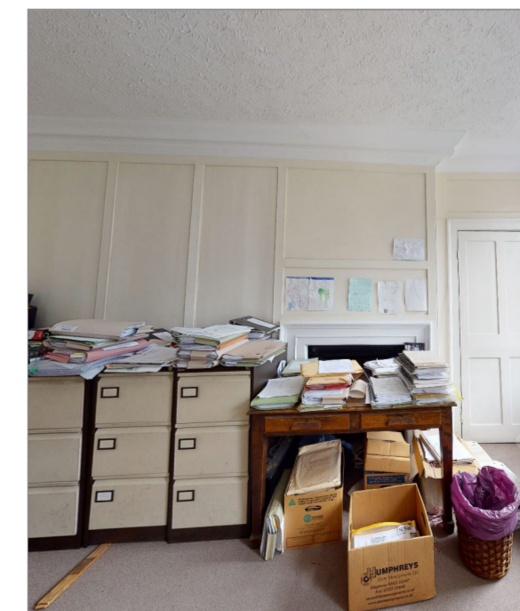
Wooden blocks used to support filing cabinets due to uneven floors Wooden
