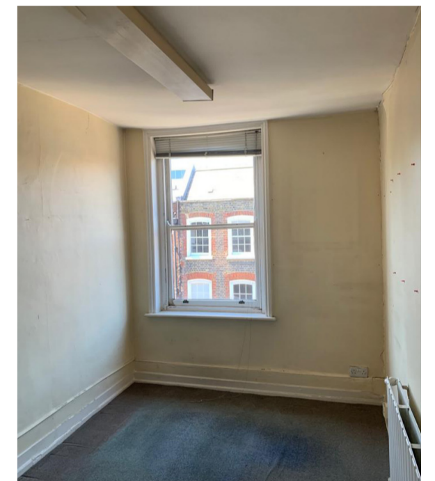
Uneven ceiling due to sagging floor joists
