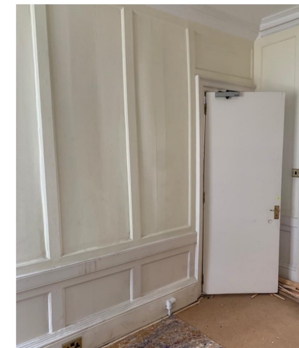
Large bowing of original timber partition
