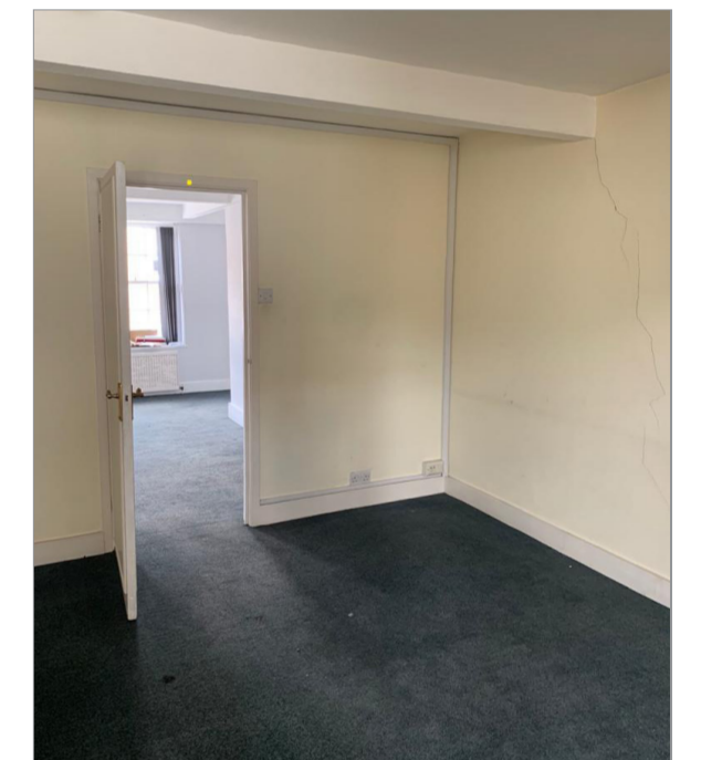
Non-original roof extension, with noticeable cracking to party wall
