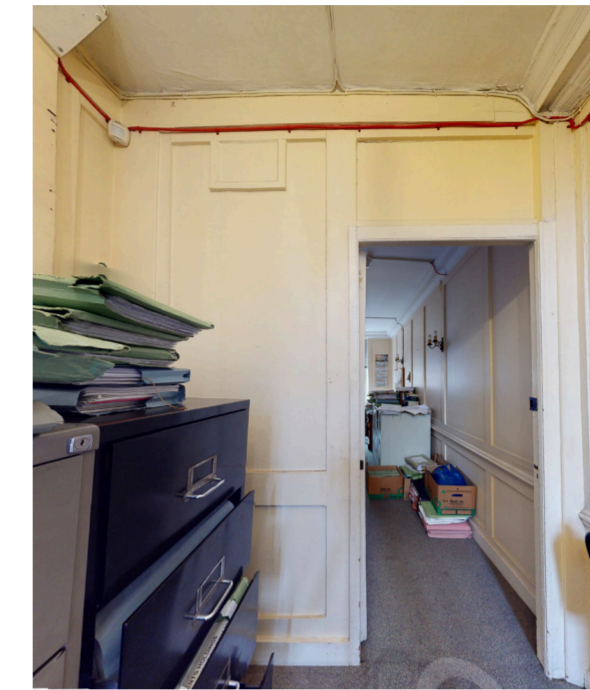
Surface mounted fire alarm cabling
