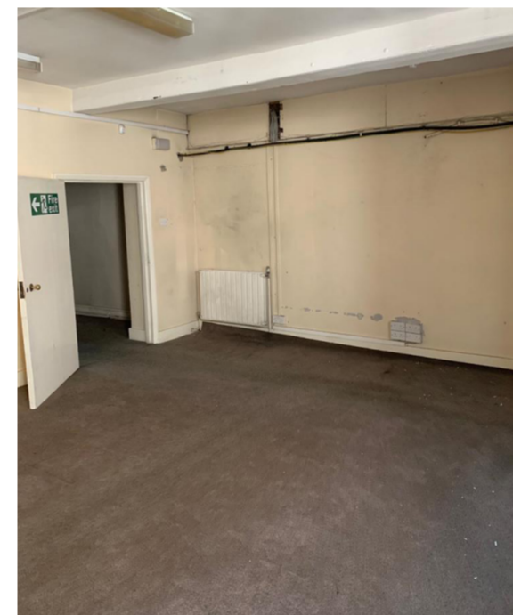
Surface mounted services throughout the property and ad-hoc fire provisions
