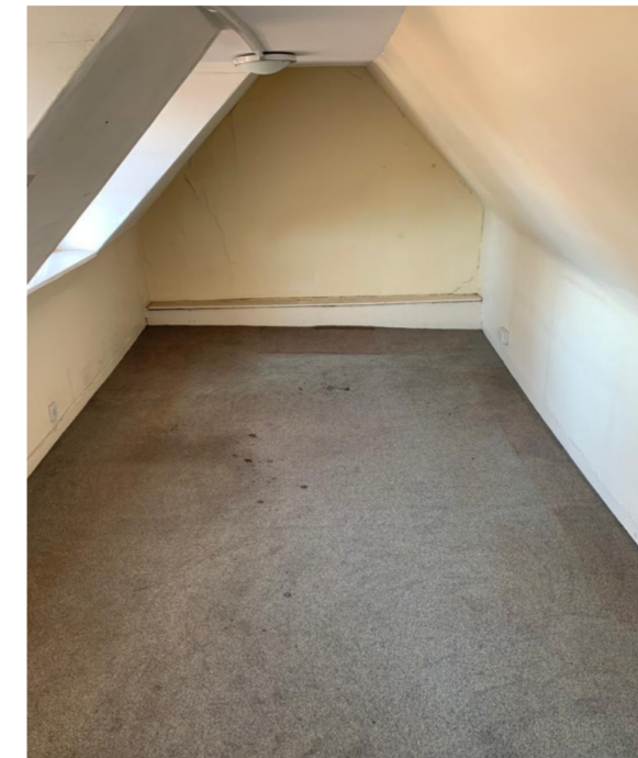
Existing loft space with compromised head height
