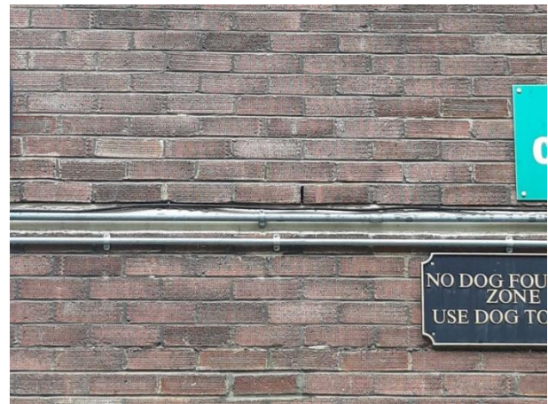
Plate 4.6: Extent of Weepholes (Building B2 - Chancellors' Court, Southern Elevation)
