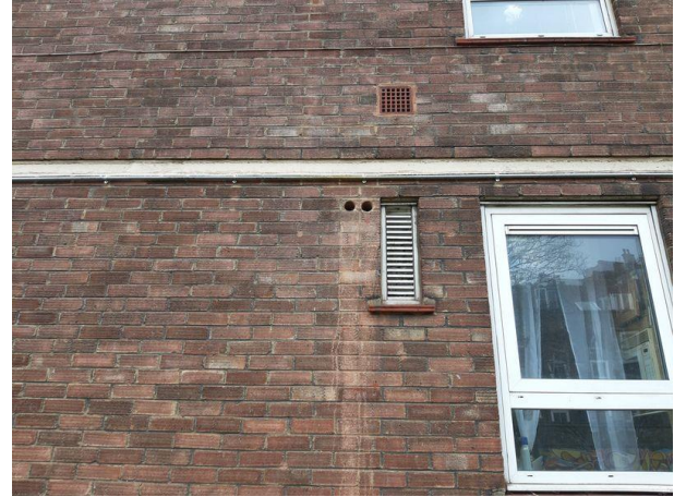
Plate 4.4: Open-ended Pipework (Building B2 - Chancellors' Court, Northern Elevation)
