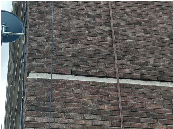
Plate 4.5: Extent of Weepholes (Building B1 - Babington Court, Northern Elevation)
