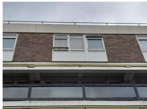
Plate 4.26: Gaps in Fascia Board (Eastern Elevation)
