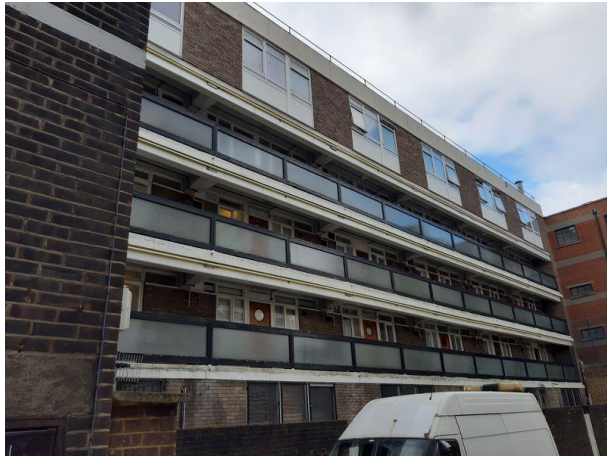
Plate 4.23: Extent of Painted Fascia Board (Eastern Elevation)
