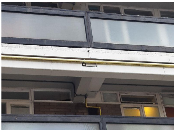
Plate 4.25: Gaps in Fascia Board (Eastern Elevation)
