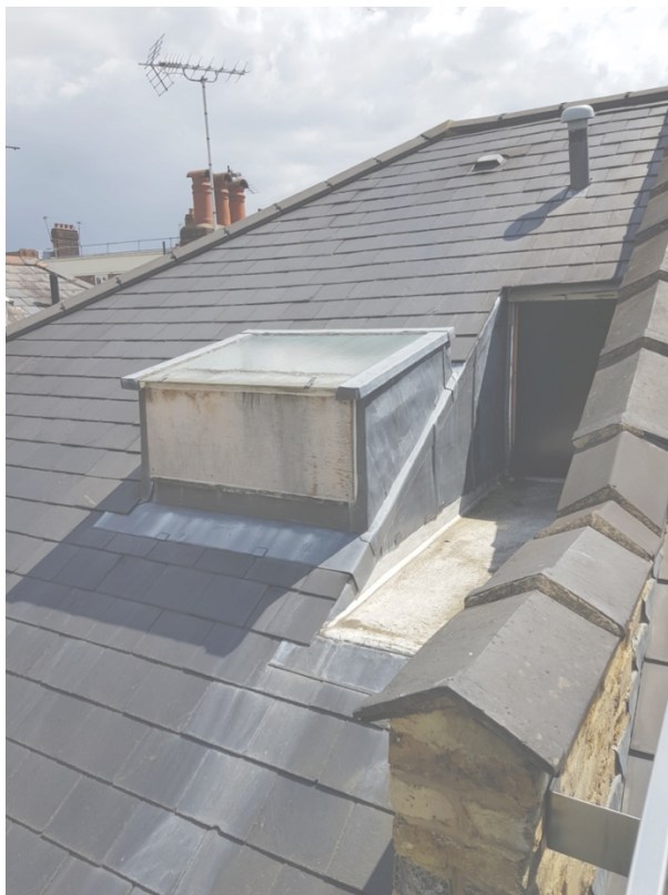
Image: View from 32 Glenloch Road looking North East illustrating roof alterations on broken symmetrical roof scape to number 30 Glenloch Road
