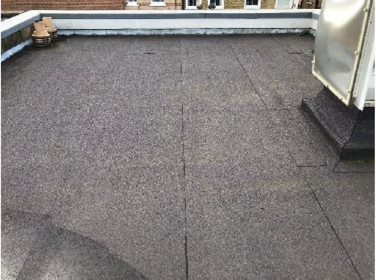
Existing flat roof and skylight. Lead capped parapet on South-west elevation also visible. This will conceal the PV panels when viewed down the street from Regents Park Rd
