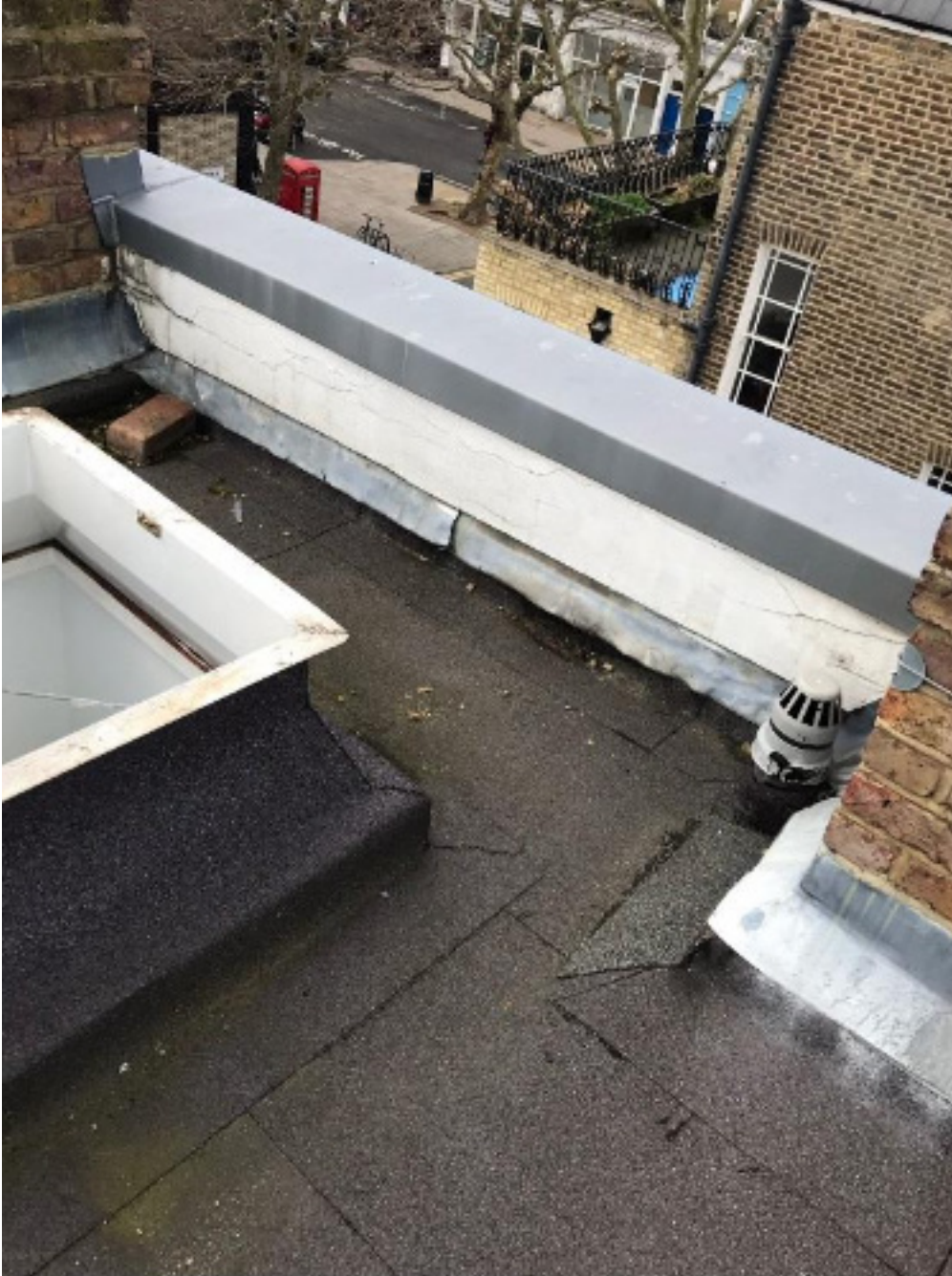
View of existing flat roof, chimneys and skylight. Lead capped parapet on North elevation also visible. This will conceal the PV panels when viewed down the street from Regents Park Rd
