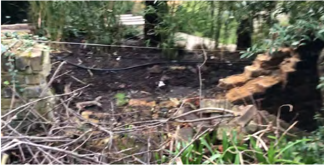
Photo 1: Collapsed section, Number 11 side
