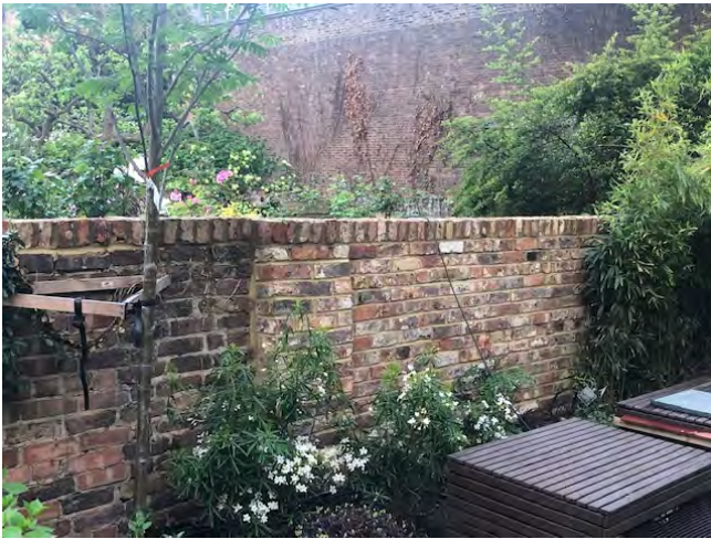
Photo 9: Junction of rebuilt wall & 2 nd pier and old recapped wall, Number 10 side
