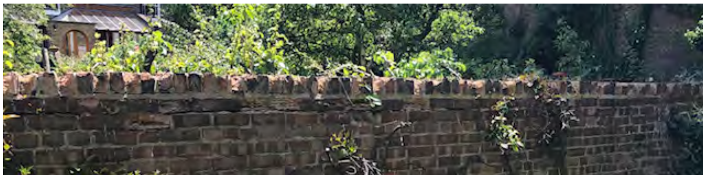
Photo 6: Condition of capping before repair
