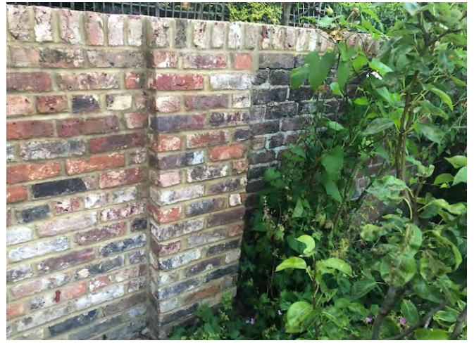
Photo 10: Junction of rebuilt wall & 2 nd pier and old recapped wall which is about 75 mm off vertical, Number 11 side
