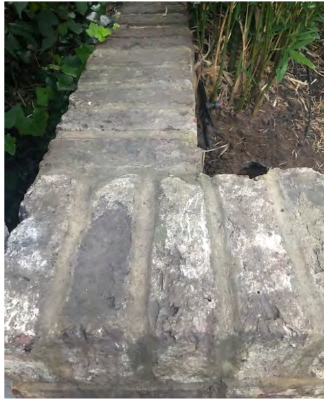
Photo 12: Junction of rebuilt wall between Numbers 10 & 11 (left to right) and existing end wall of Number 10 (top to bottom)
