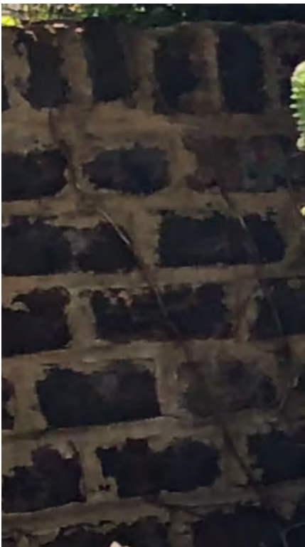
Photo 5: Old cement repairs, Number 10 side
