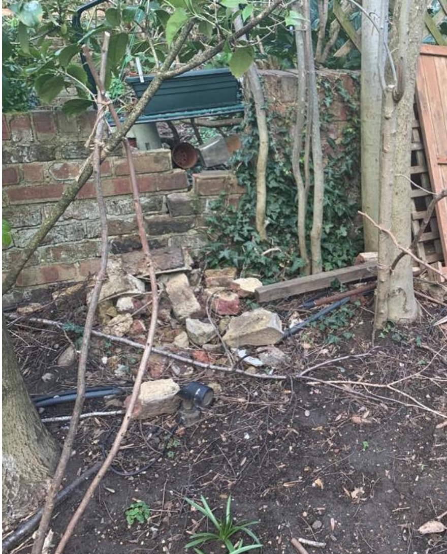
Section of wall cracked / crumbling due to tree roots nearby.
