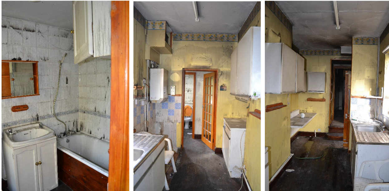
Fire damage to the ground floor flat bathroom and kitchen prior to conversion back to a family dwelling
