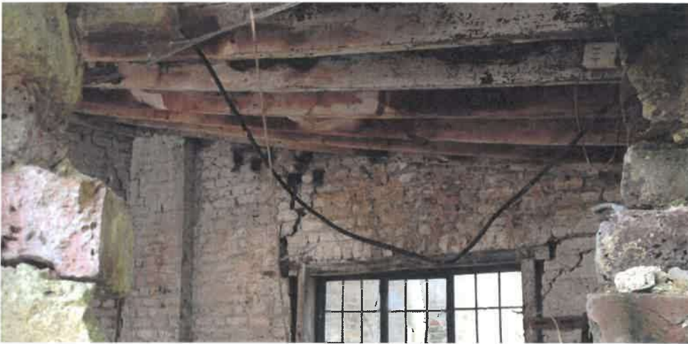
Decaying roof timbers, likely caused by water ingress.
