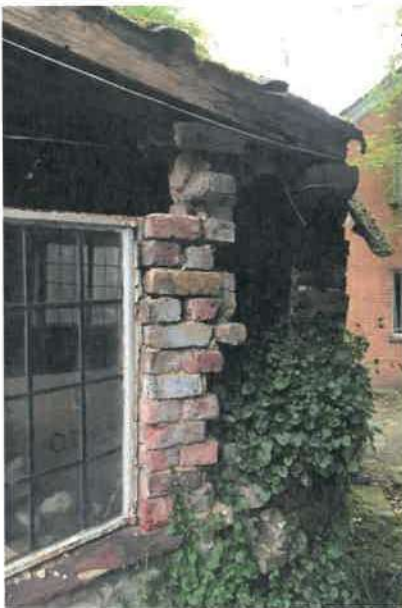
South-east view of existing external wall, showing large areas of missing bricks, cracks and bowing.
