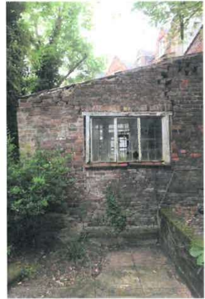
View to north-facing external wall- showing severe cracking and damage.
