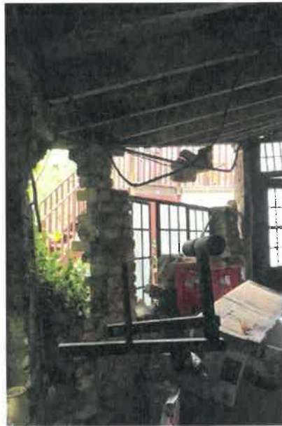
Internal view looking south, the existing roof supported by an insecure brick pier.
