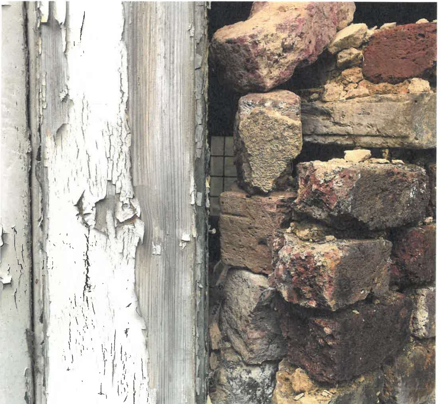
EXISTING OUTBUILDING WALL CONDITION
