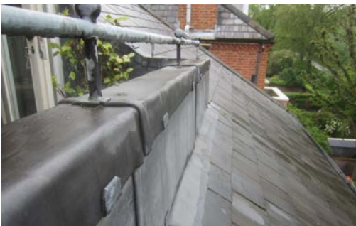
Lead detailing to rear roof terrace as existing Note: Lead fascia and capping with wetted joints to be replicated in proposed alteration.
