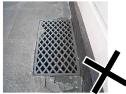
Grille – not acceptable
