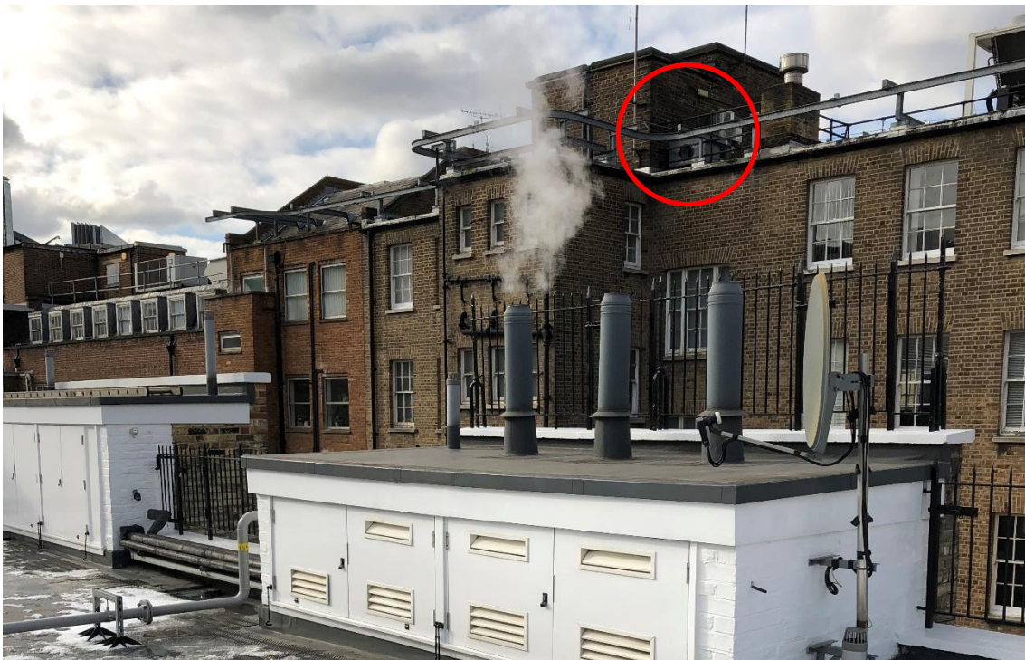
Figure 5 Noisy fan on rooftop of Ely Place
