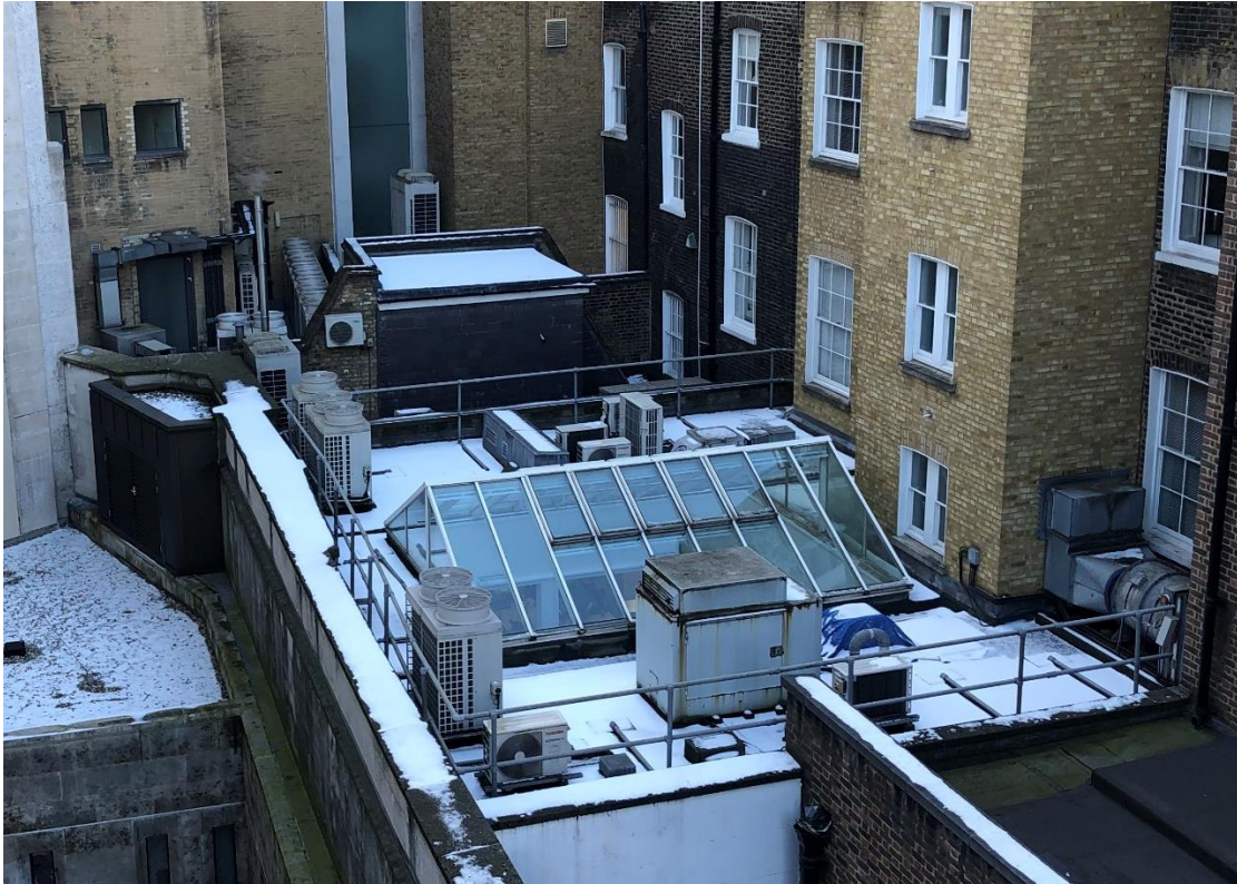
Figure 6 Plant equipment on the Ely Place rooftops to the south west of position 2
