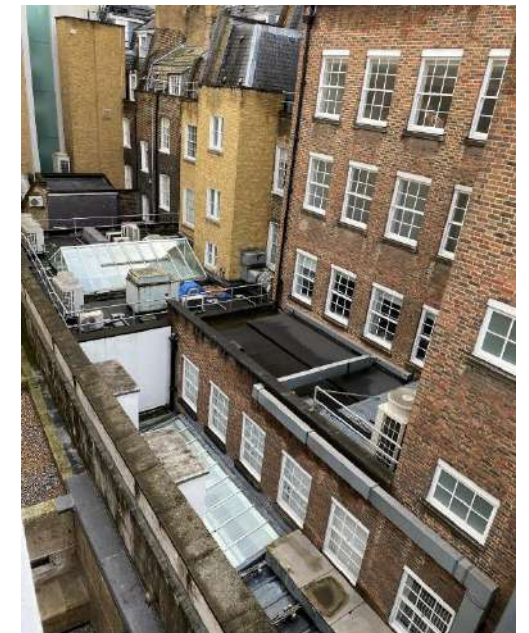
VIEW OF THE REAR OF THE ELY PLACE BUILDINGS, TAKEN FROM THE ROOF OF ST ANDREWS HOUSE LOOKING SOUTH-WEST.
