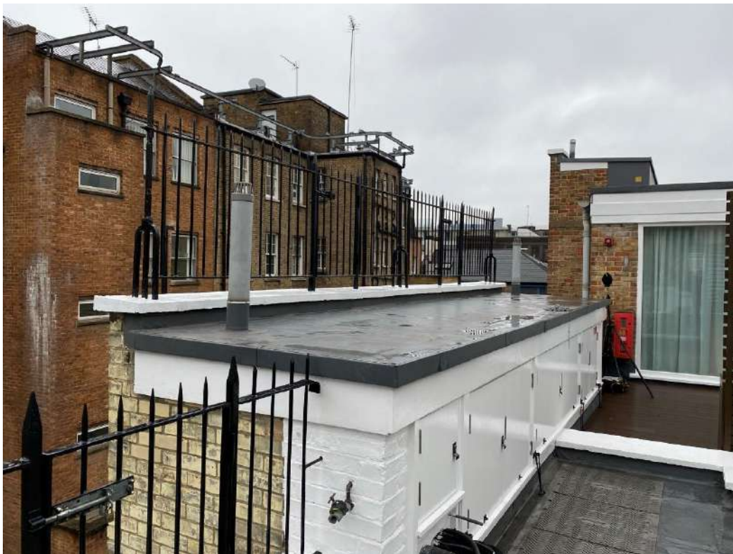
FORMED IN BRICK WITH A SIMPLE ROOF, EACH OF THE PLANT ENCLOSURES – BUT ONE – ARE TOPPED IN EXISTING CAST-IRON RAILINGS
