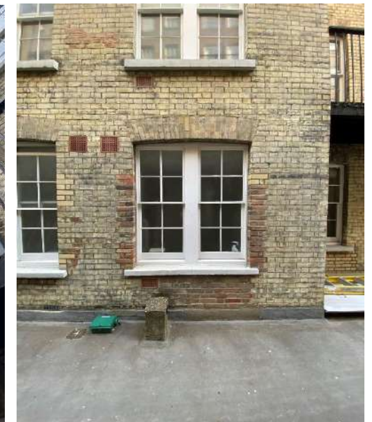
ALONG THE REAR, AT LOW LEVEL, ARE A NUMBER OF NOW REDUNDANT CONCRETE GAS-PIPE MOUNTS
