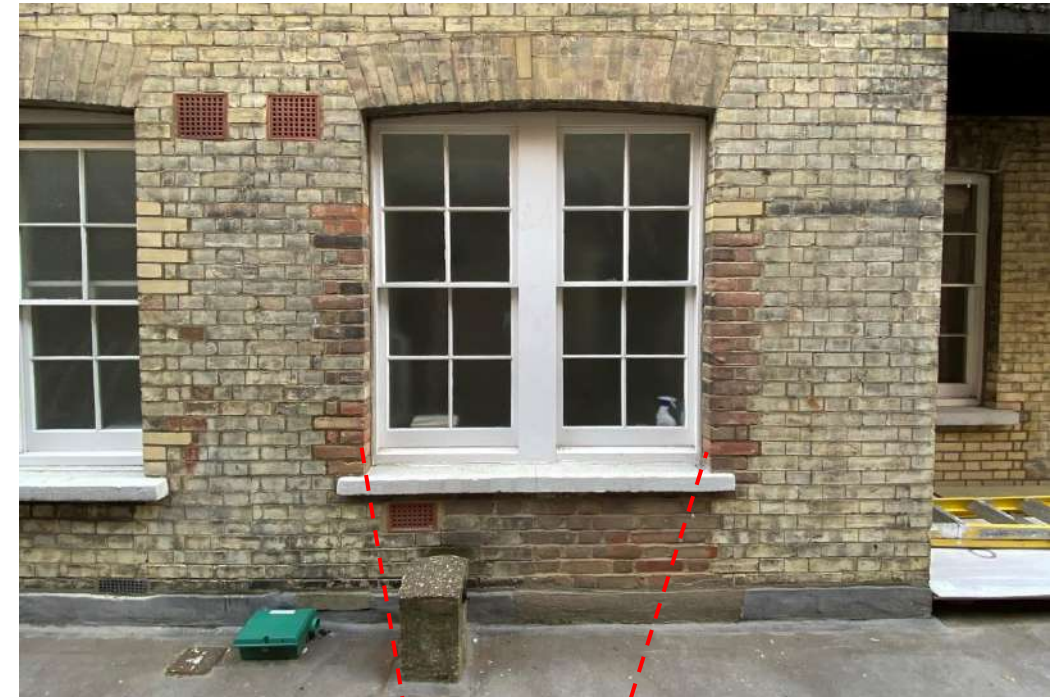
EXISTING REAR WINDOW WILL BE MODIFIED TO BE A NEW SERVICE DOOR. EXISTING EXTERNAL FEATURES WILL BE REMOVED
