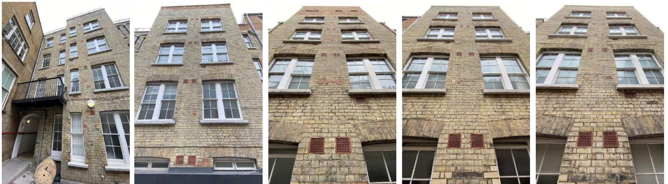
THE REAR (WEST) FAÇADE HAS BEEN REPAIRED AND CLEANED A NUMBER OF TIMES OVER THE YEARS, HOWEVER, THE WINDOWS ARE LARGELY ORIGINAL. TERRACOTTA AIR-BRICKS ARE SET OUT IN BAYS, ORIGINALLY USED FOR GAS VENTING AND VENTILATION.
