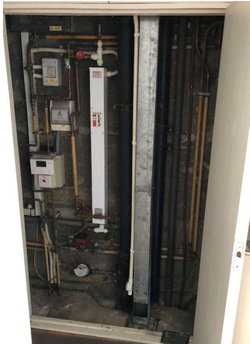
Fig C.1 – Typical riser cupboard in lower level of apartments showing duct from below to above
