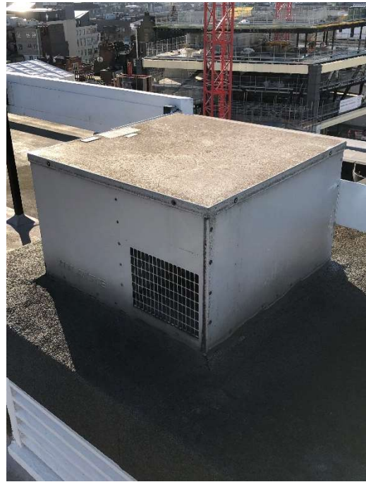
Fig C.4 – Typical communal extract fan
