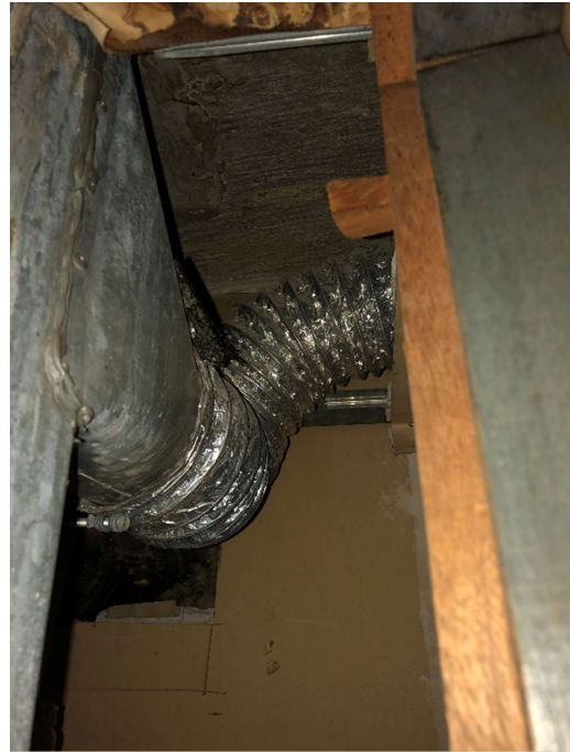
Fig C.2 – Typical branch off common duct in upper level water tank cupboard, enter landing ceiling void
