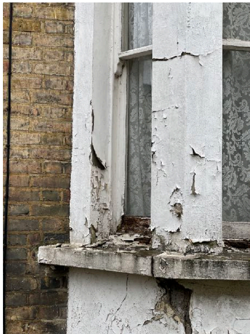
Destroyed window cill profile on the front of No 63
