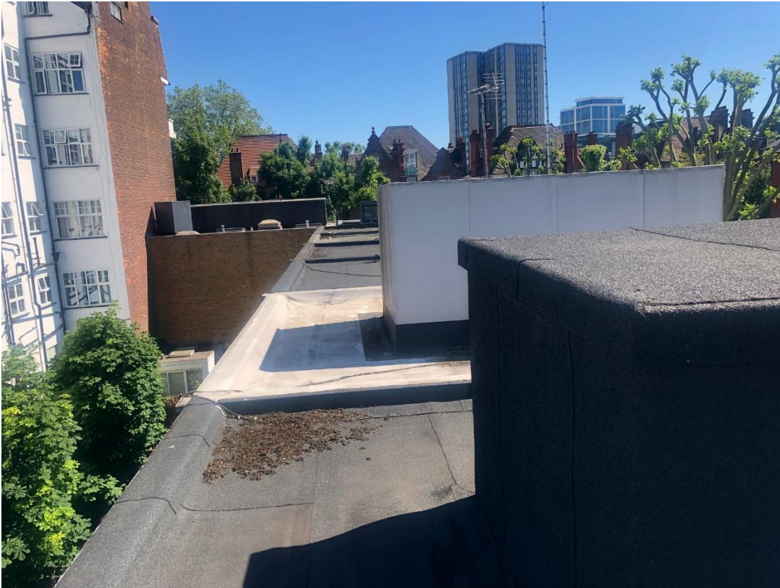
5. 25 Crossfield Rd roof looking towards 26 with 52 and 50 Eton Ave at the end
