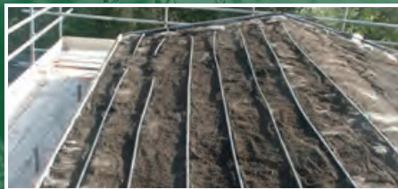
■ Drip irrigation kit installed
