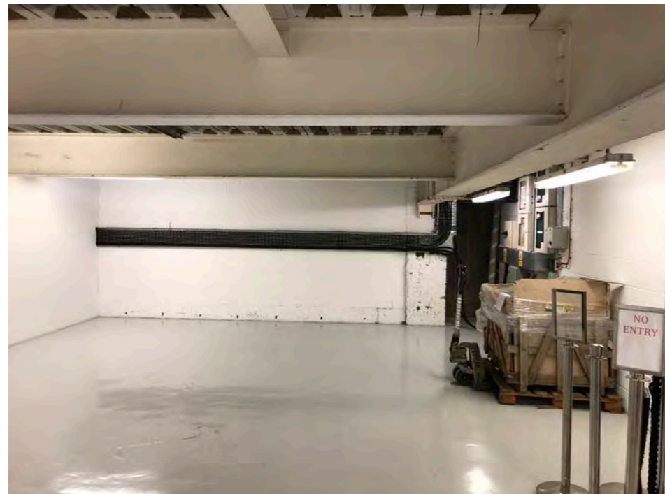
Area of proposed changing rooms. 40mm screed to be removed to increase headroom.
