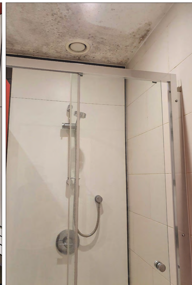
Existing shower cubicles and ceiling to be stripped out, extraction issues to be addressed
