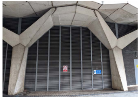
Site photo - existing 33kV UKPN substation louvred facade.
