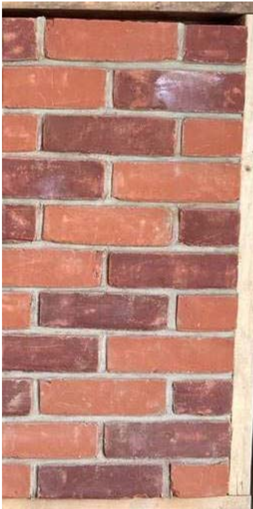
Revised pointing sample – ' Slightly recessed pointing '
